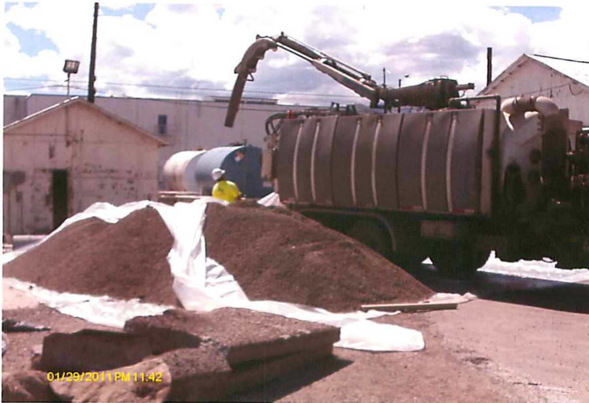
This picture shows the contaminated stockpile. This picture was taken looking in a westerly direction.
