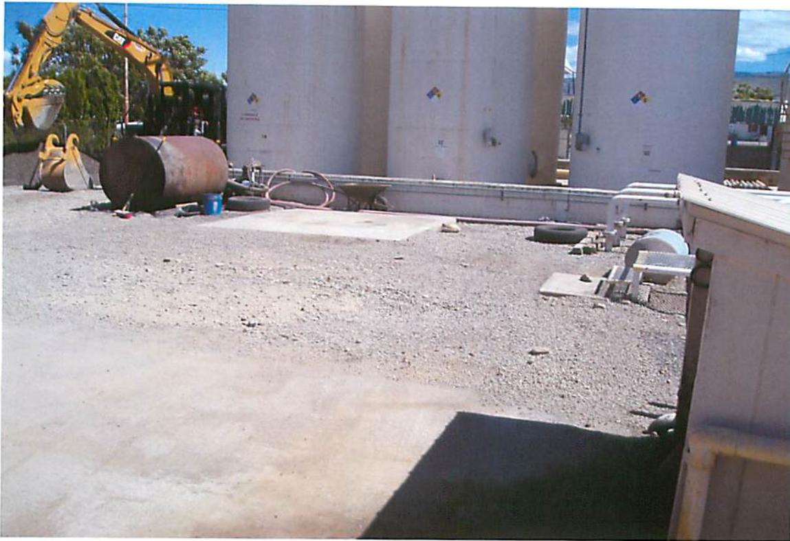
This picture shows the stockpile area after removal of the contaminated soils and plastic. This picture was taken looking in a southeasterly direction.
