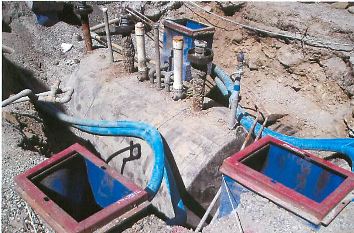
This picture shows the continued vacuuming process and the UST. This picture was taken looking in a northerly direction.
