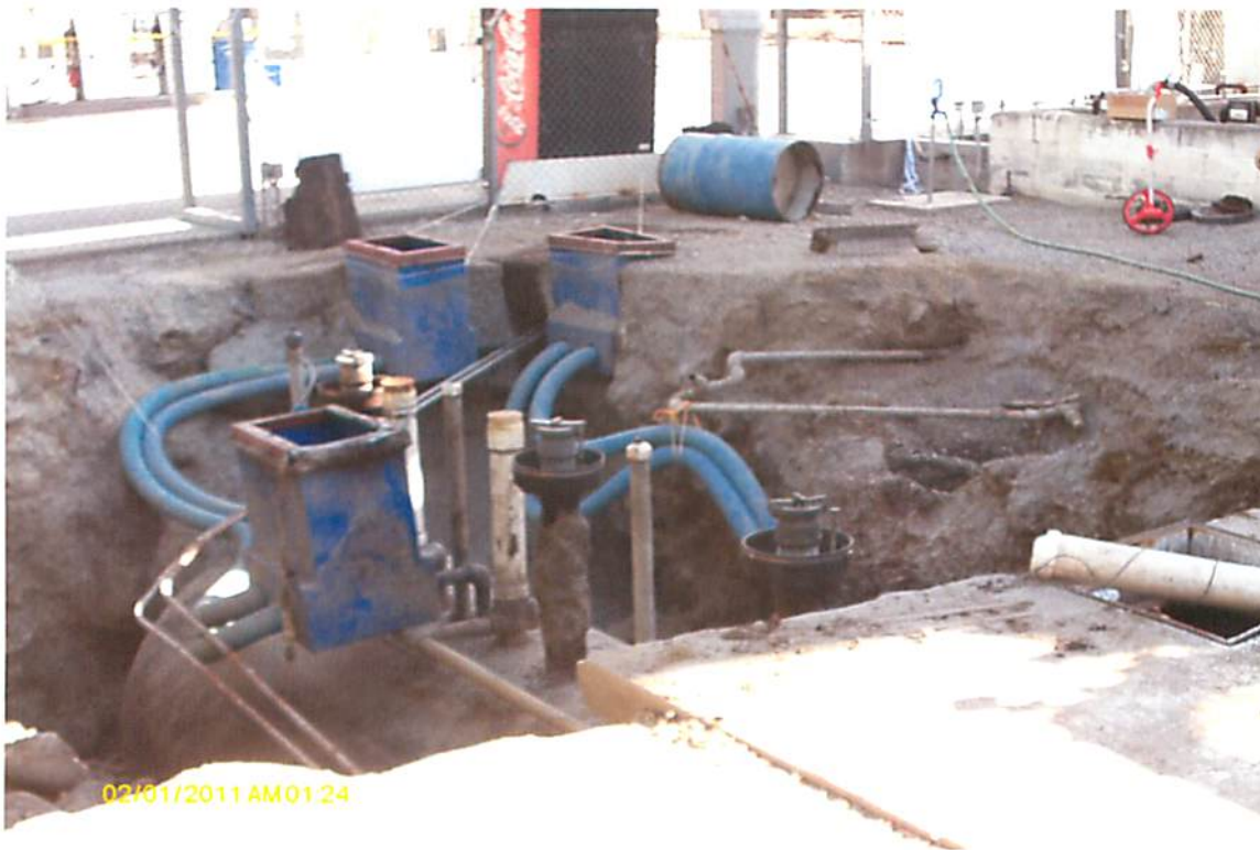
This picture shows the excavation process and the exposed UST. This picture was taken looking in a southerly direction.
