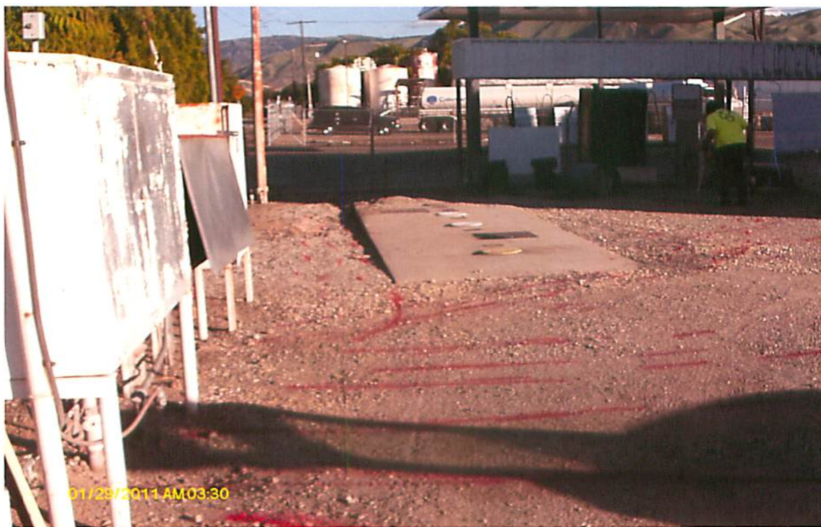
This is the site when ACT first arrived. Note the red lines denoting underground utilities. This picture was taken looking in a southeasterly direction.
