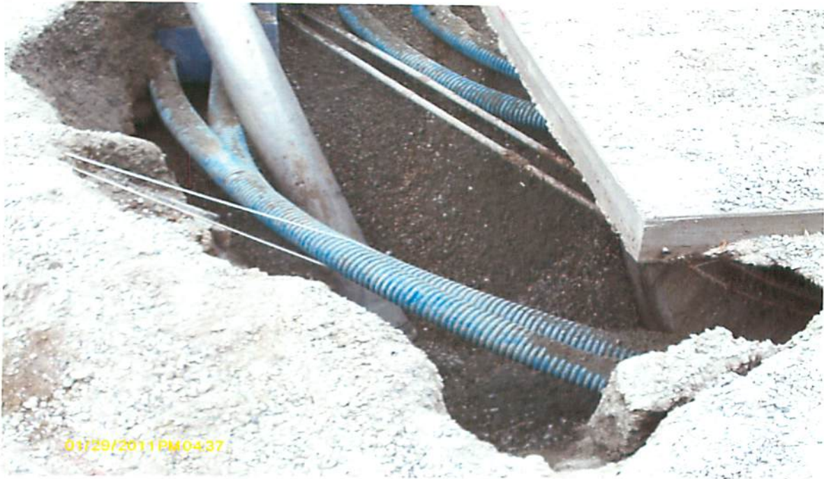
This picture shows the vacuuming process and the product lines. This picture was taken looking in a southwesterly direction.
