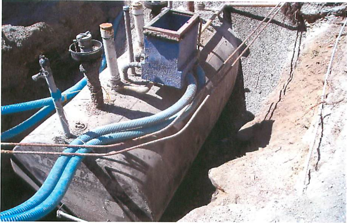
This picture shows the excavation and the UST. This picture was taken looking in a northwesterly direction.
