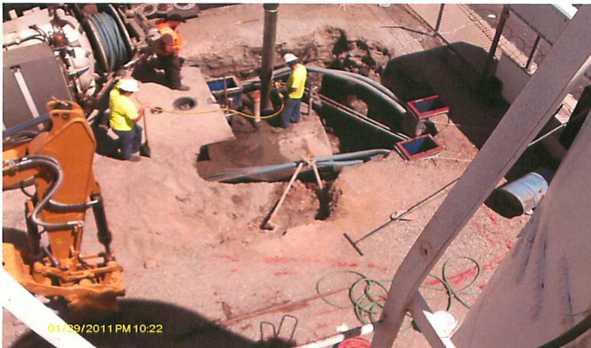
This picture shows the continued vacuuming process and the UST. This picture was taken looking in an easterly direction.
