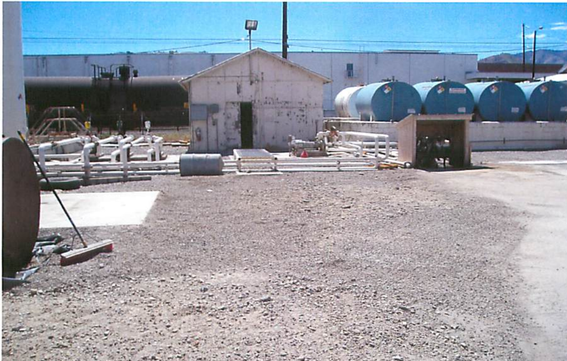
This picture shows the stockpile area after removal of the contaminated soils and plastic. This picture was taken looking in a southwesterly direction.
