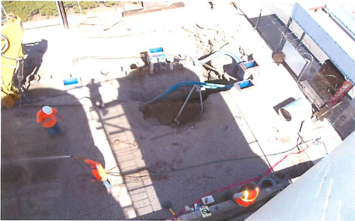
This picture shows the finished excavation and the UST. This picture was taken looking in an easterly direction.
