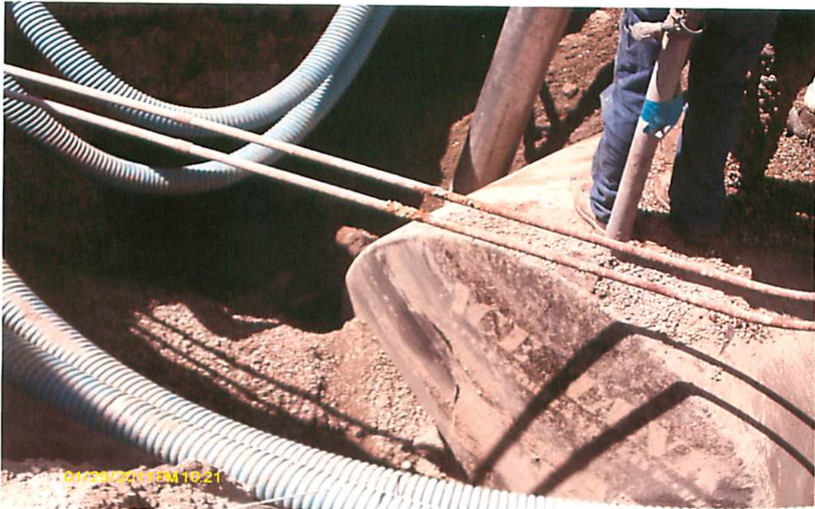
This picture shows the continued vacuuming process and the UST. This picture was taken looking in a westerly direction.
