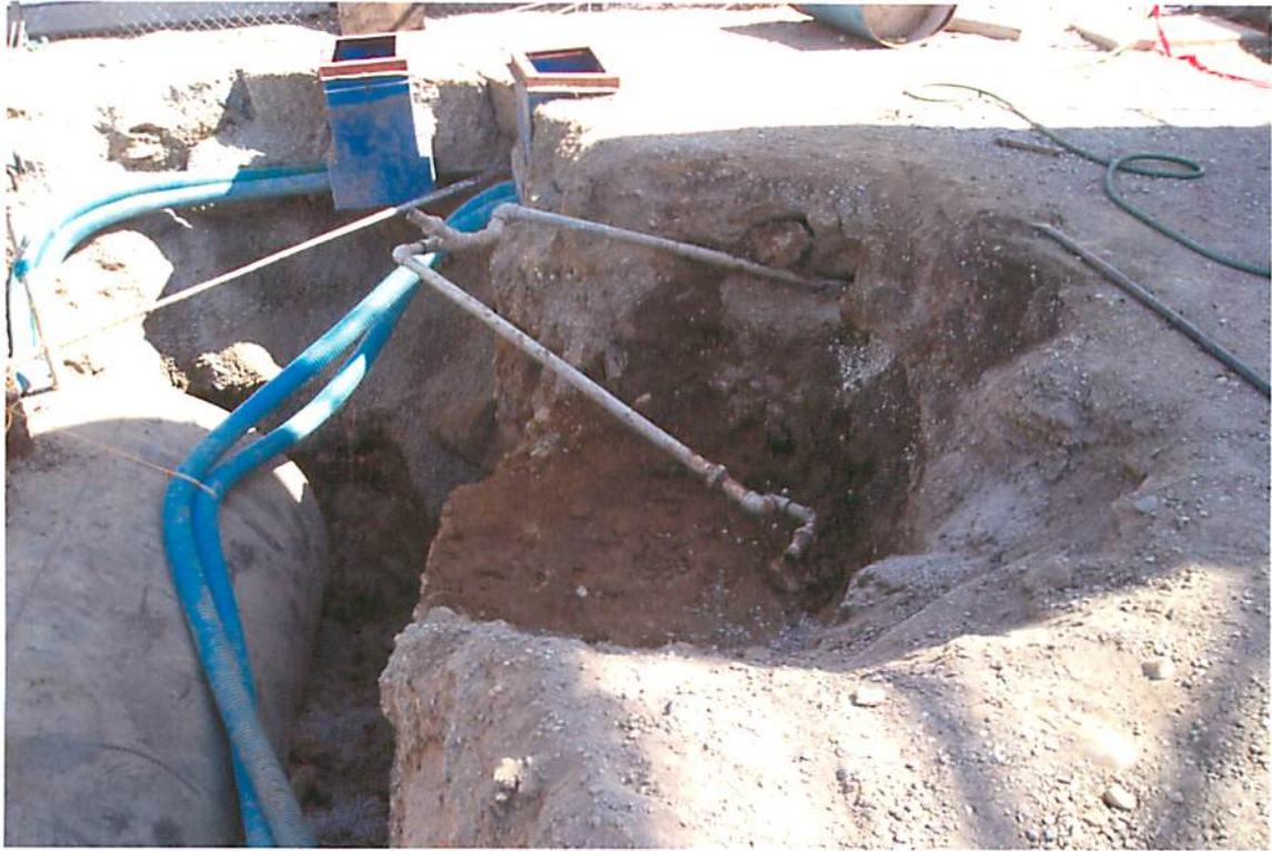
This picture shows the additional excavating process and the UST. This picture was taken looking in a southeasterly direction.
