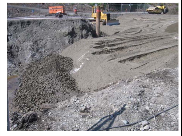
Photo 6. Backfilling Area A excavation looking northwest. Suitable re-usable onsite soil on the bottom (darker) and clean imported material on the top (lighter).
