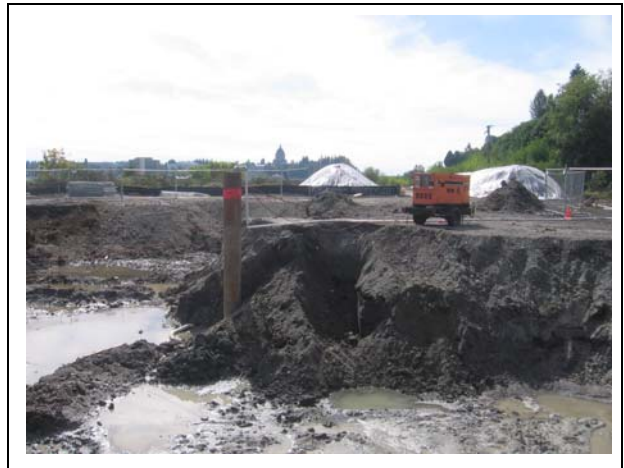
Photo 4. Entire excavation open after extra excavation overseen by Ecology has been completed. Covered stockpiles of segregated excavated material from Area A can be seen to the south in the background.
