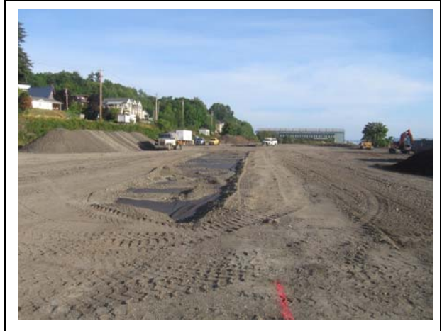
Photo 14. Area C looking north after rail removal, excavation, and geotextile marker installed.
