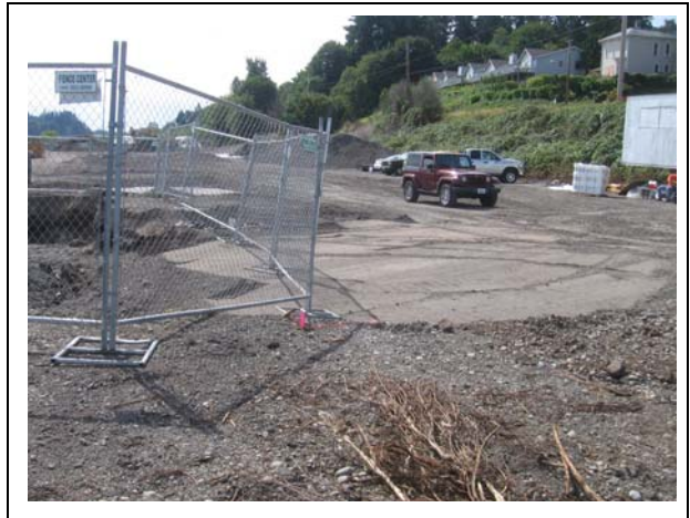
Photo 12. Backfilled Area B to the west and additional excavation to the east.
