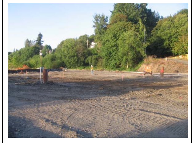
Photo 2. Area A after clearing and grading just prior to start of remediation looking southwest.
