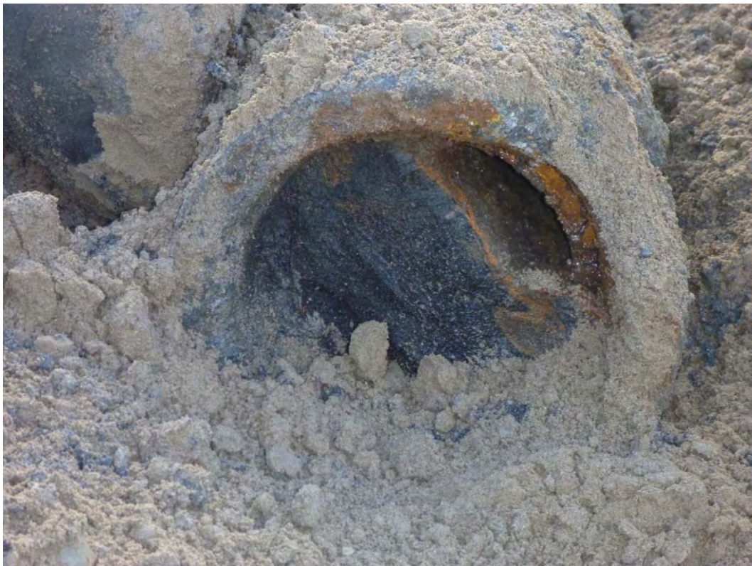
Photograph 14. Sandblast Grit Encountered in Former Storm Drain Pipe.
