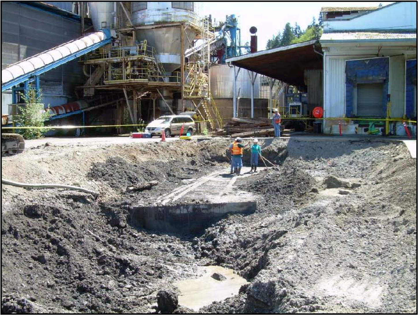
Figure 2-6 Subsurface Concrete Structure, May 2006 Remedial Investigation/Feasibility Study Abitibi West Tacoma Mill Steilacoom, WA
