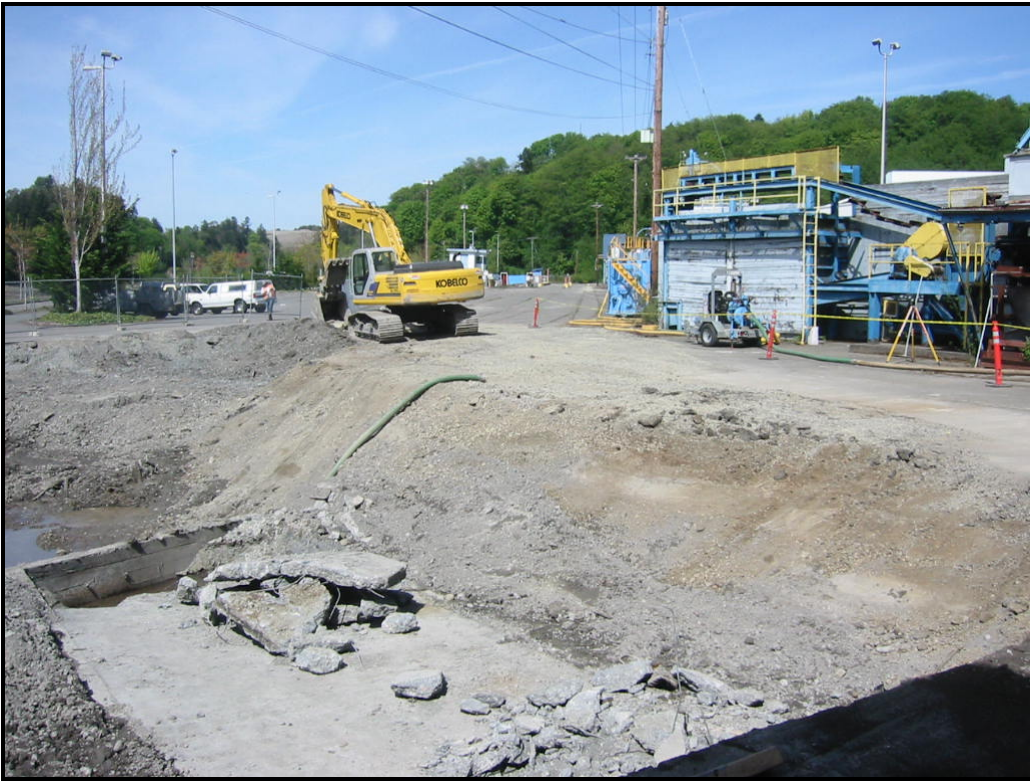
Photo 3. Concrete structure of unknown origin, 5-6 feet below ground surface.
