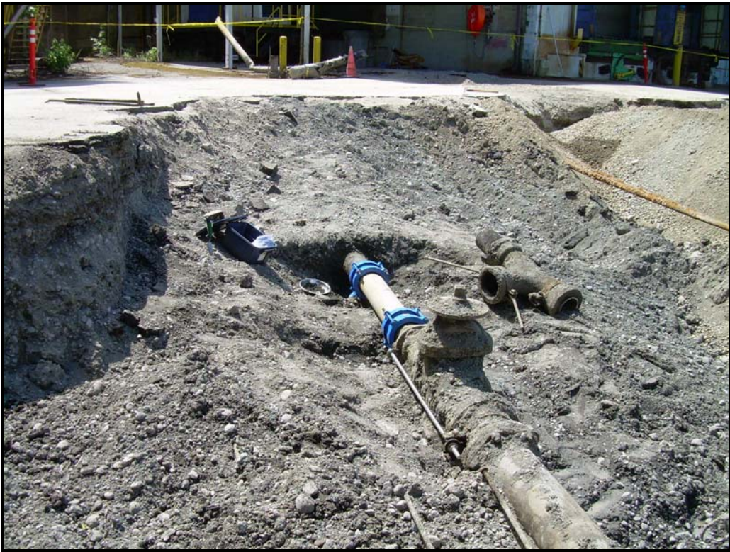
Photo 4. Eight Inch ductile iron fire water control line, four feet below ground surface.
