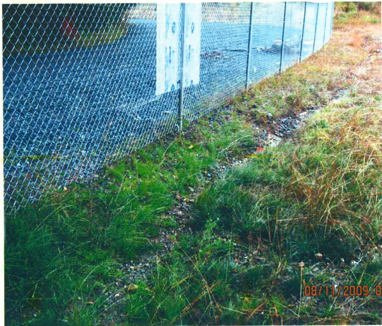
A Avenue Landfill SHA Photos – view of drainage ditch along south side photos by Polly Dubbel
