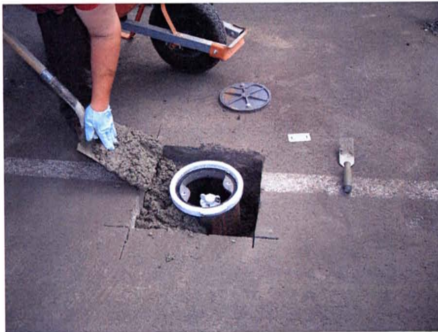
Photograph No. 4: View of groundwater monitoring well MW-01 completion.
