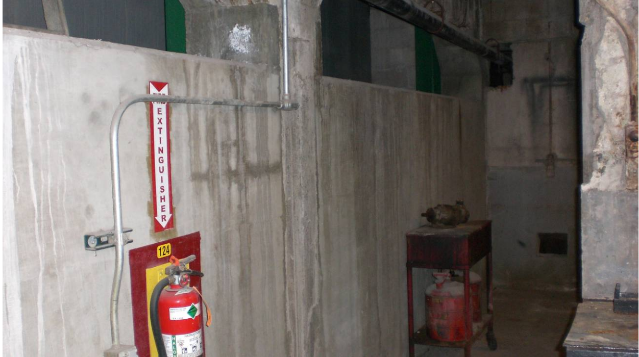
Photo 3: New Tank Location within Secondary Containment - from the northeast
