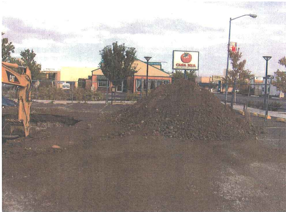
Photo 2: Photograph of removal of soil backfill (overburden) from July 2005 interim cleanup event at beginning of second remedial excavation.
