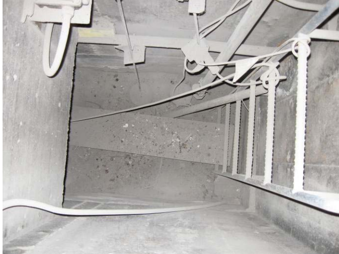
Photo 1 AOD Pit (Dry)
