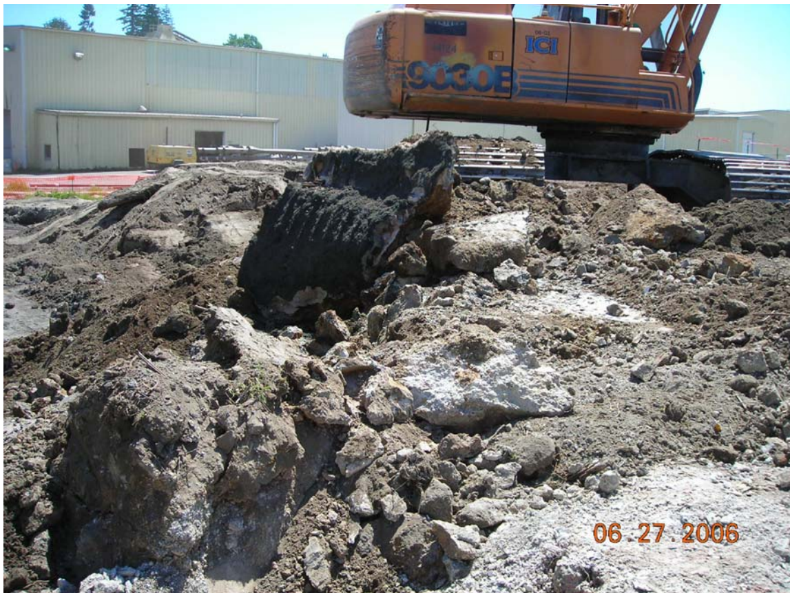
I-5, pieces of concrete-like material, looking southeast.
