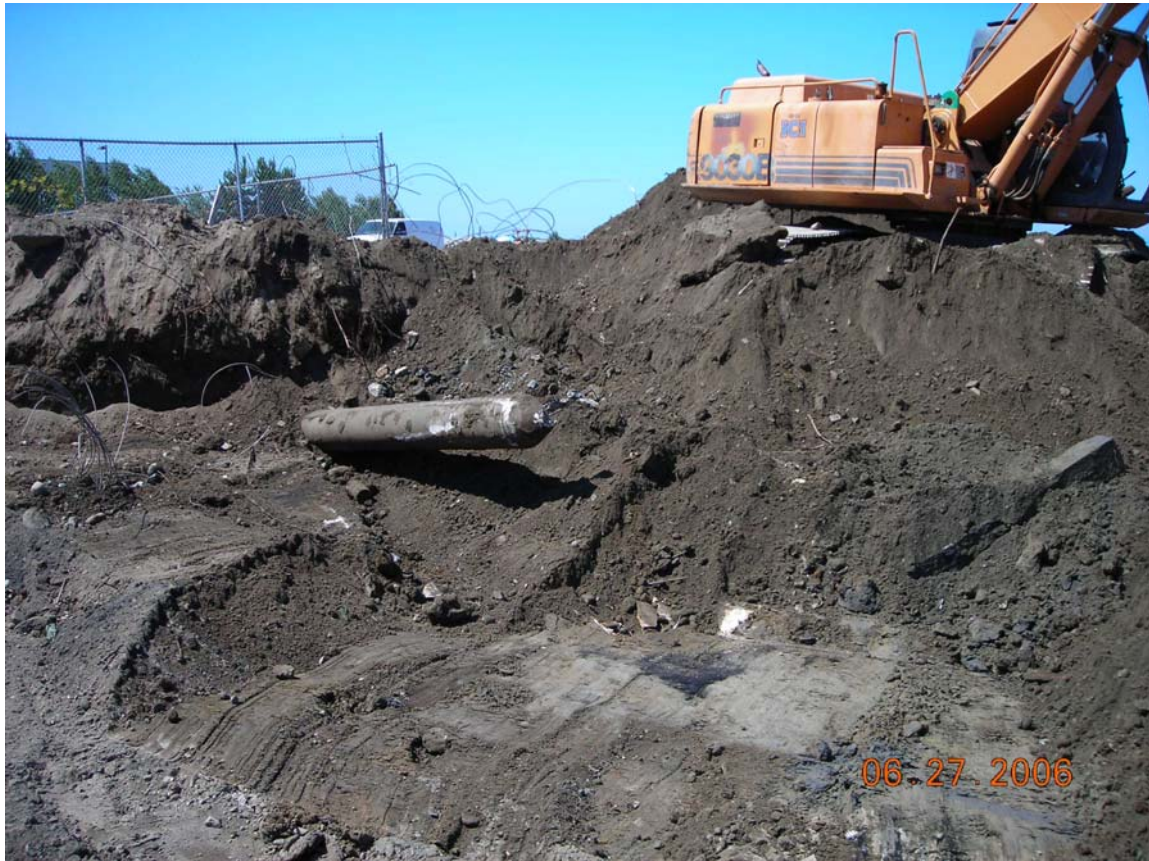
Concrete pole debris at south end of G-1, looking SW.
