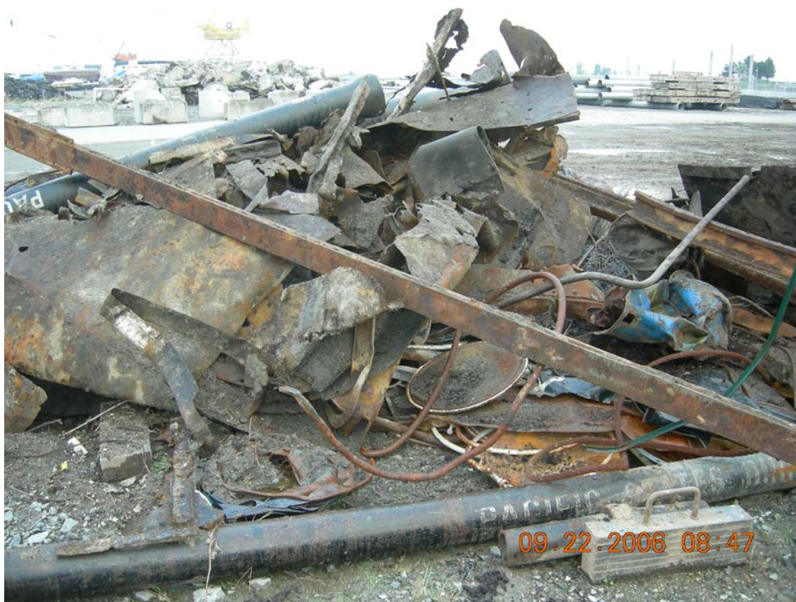
Metal debris removed from J-1 chambers.
