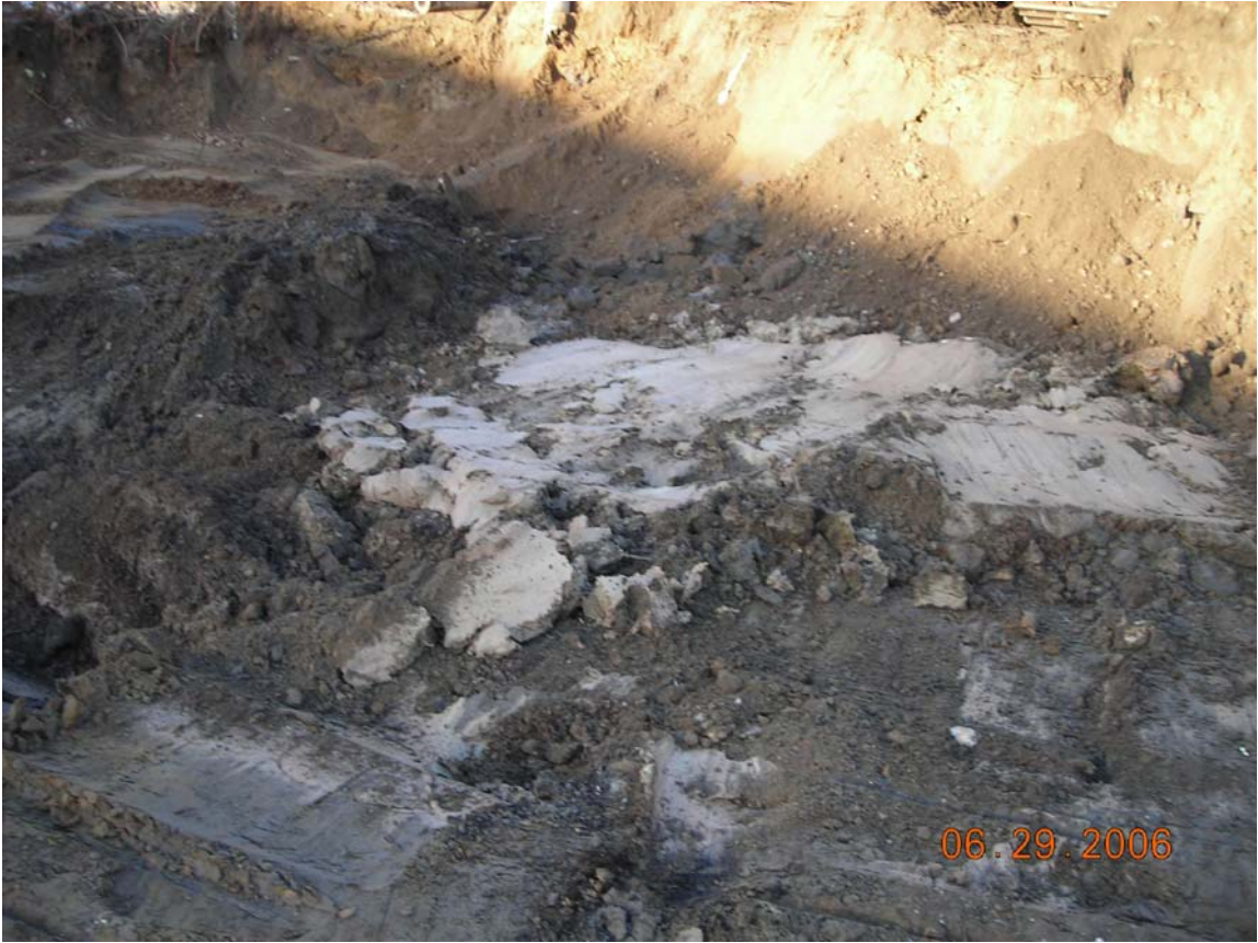
Concrete-like mud at south end of G-1.
