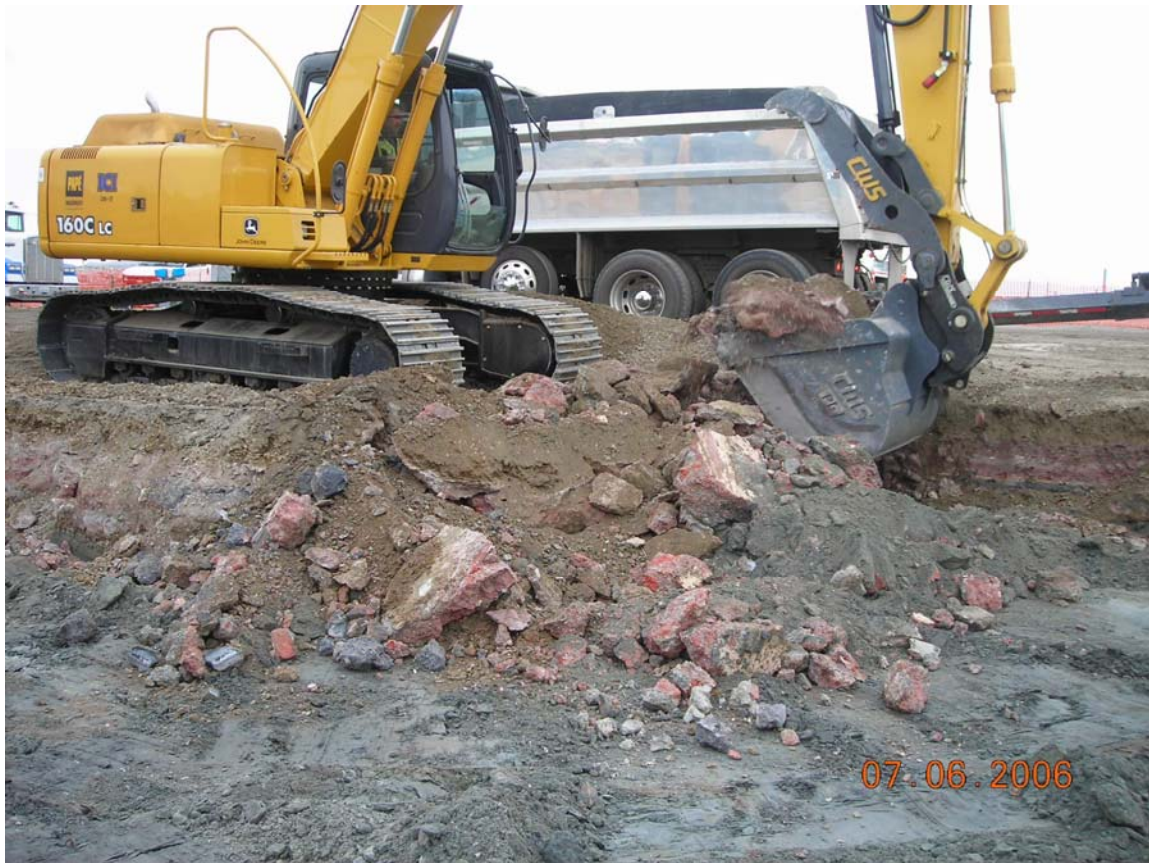
Colored concrete-like material along I-3a and I-2 boundary.
