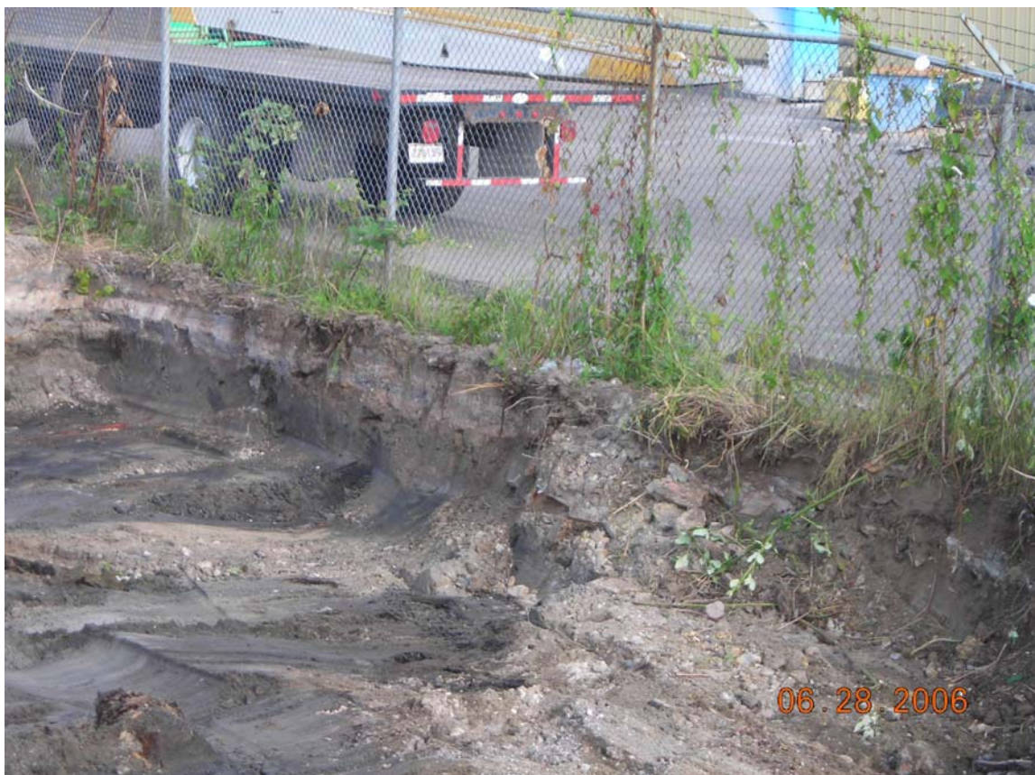
Concrete-like material layer extending under north fence of I-5 at eastern end, looking north.
