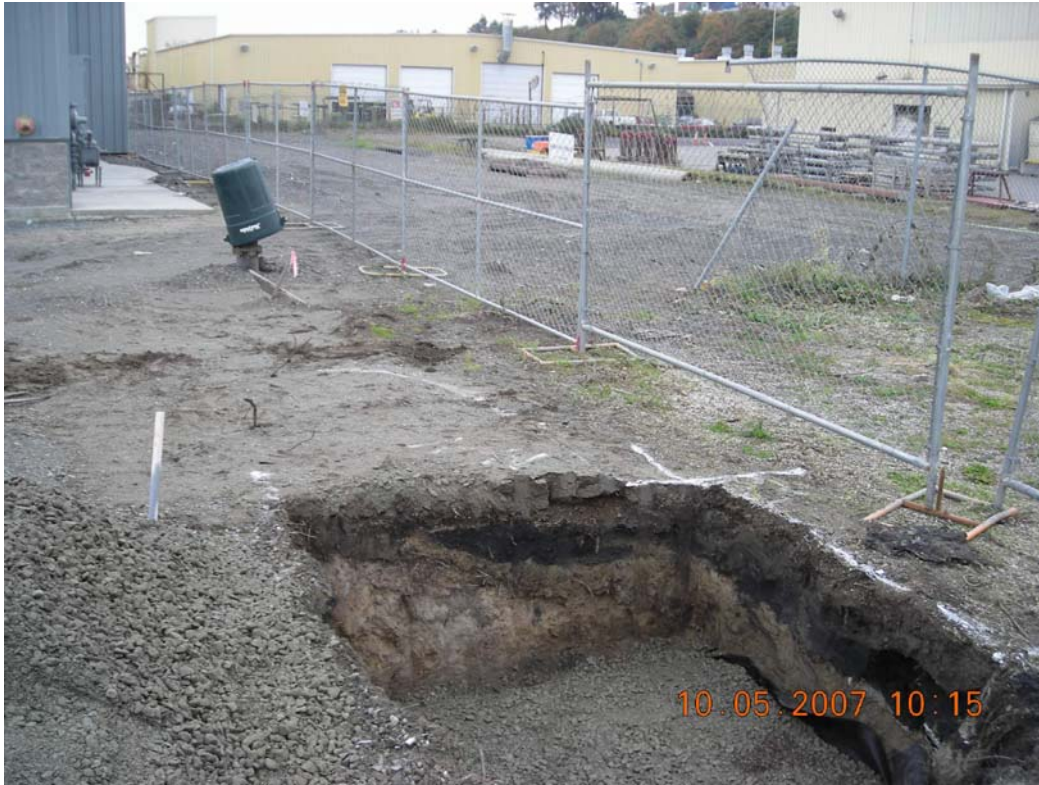
G-1a, looking north northeast before start of excavation. Note black sand material.
