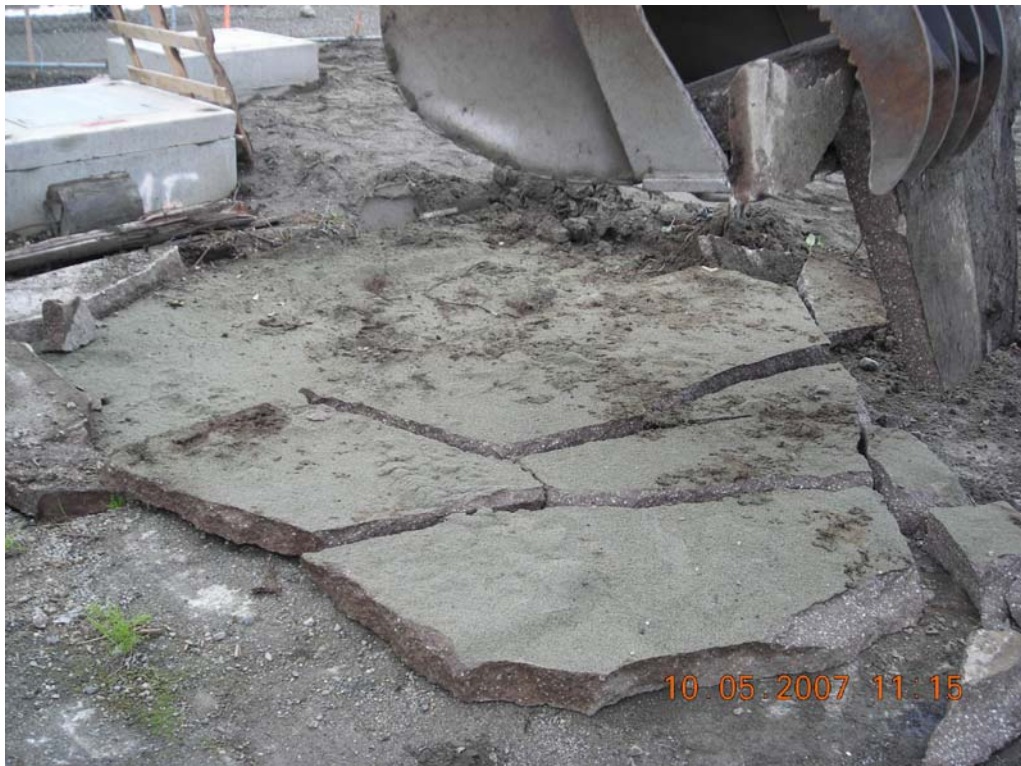
G-1a, looking southwest at purple concrete slab that was removed to access cleanup area.
