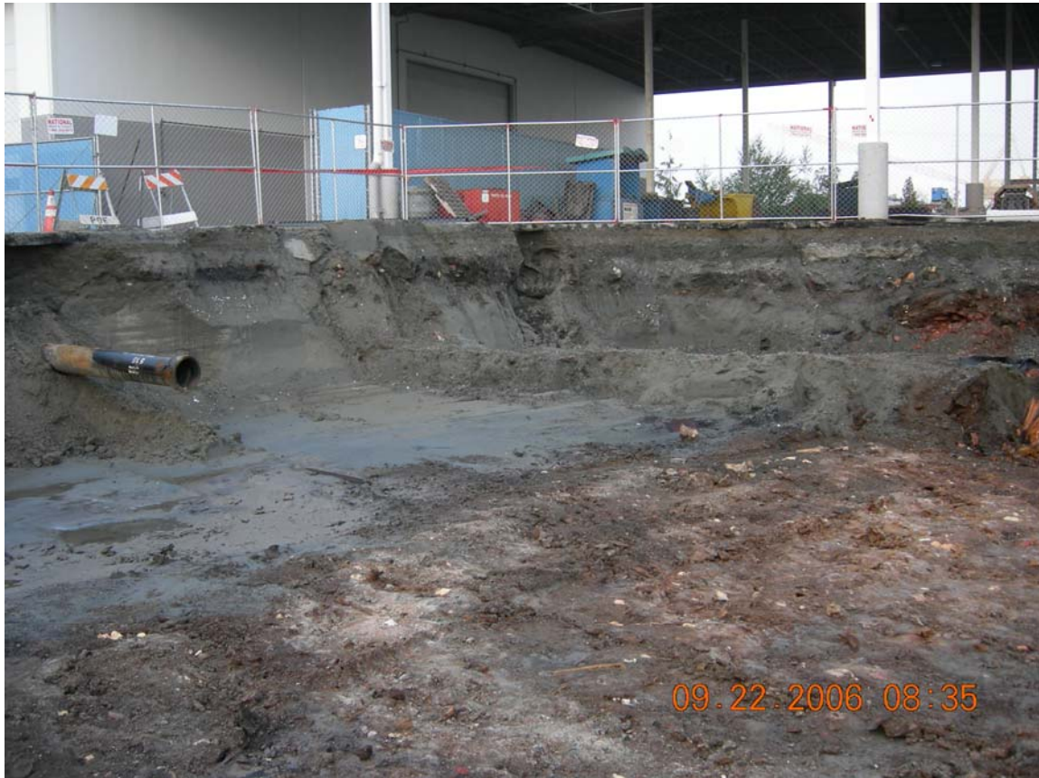
J-3, looking southwest at south edge of construction debris.
