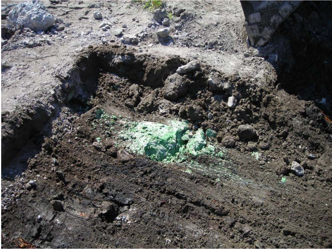
G-1, Additional excavation material west of area with desiccation cracks.
