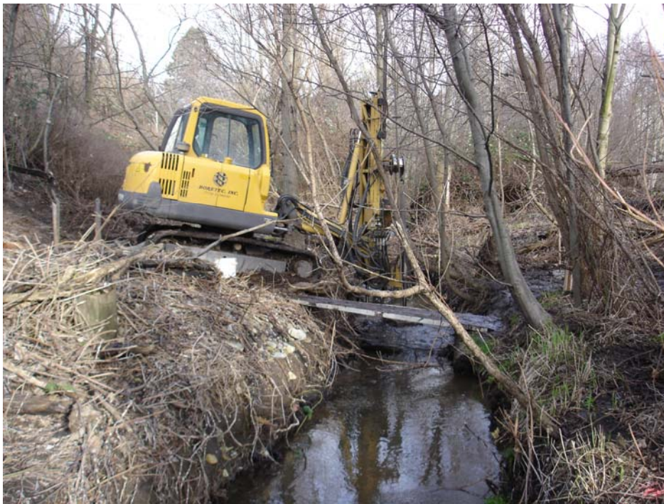
Photo 8. Track-mounted hollow-stem auger drill rig used to advance soil borings and install piezometers. Soil boring station SB-5 is shown in the photo.
