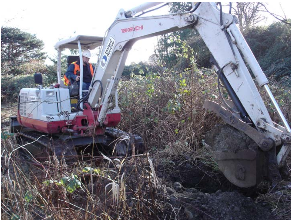
Photo 6. Small track excavator used to excavate test pits. Reconnaissance test pit RTP-13 is shown in the photo.
