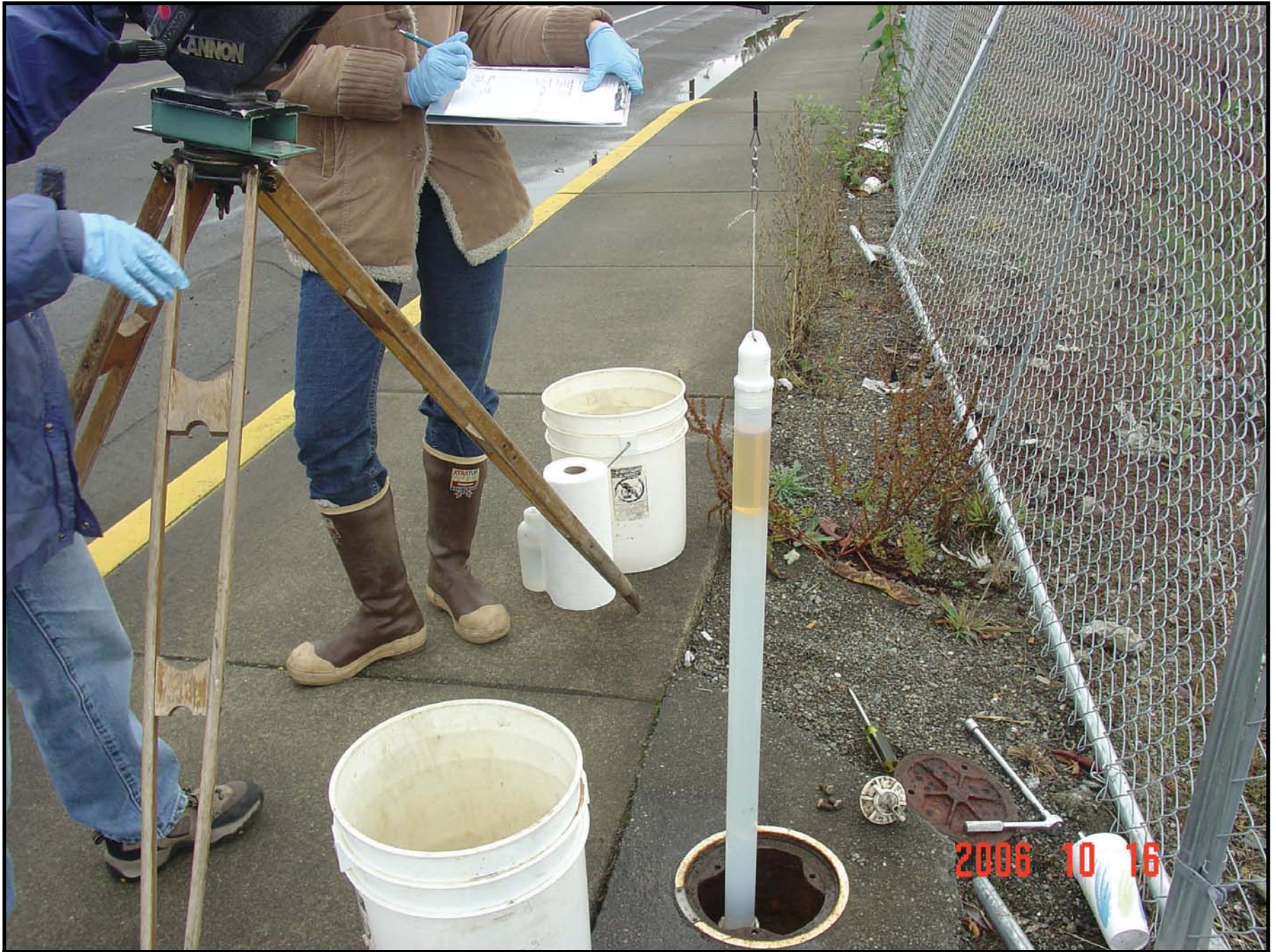
Figure 9. Sampling with bailers in monitoring wells that contain free product.
