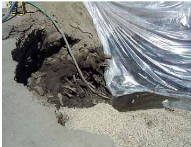
Photo 6 Backfill, dewatering accomplished with portable pump, note size and type of wood debris
