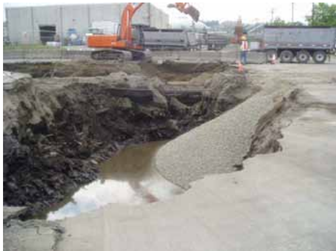
Photo 5 Backfill, note crushed rock placed in excavation providing erosion control and confinement of cut slope
