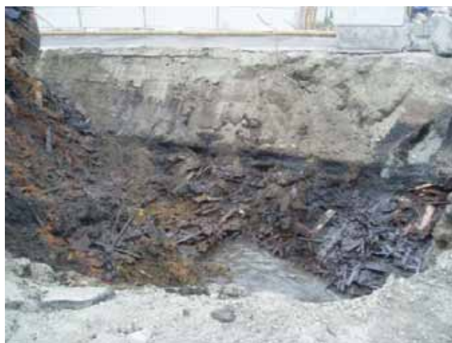
Photo 4 Wood debris, note water approximately 10 feet below ground surface (jersey barrier for scale)
