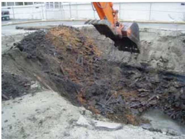
Photo 3 Wood debris, note thickness of soil fill and size of wood debris
