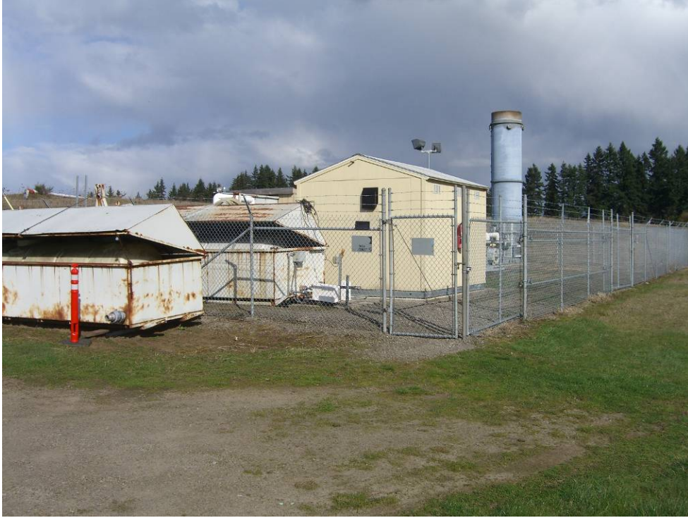
Photo 1: South Flare – from the west
