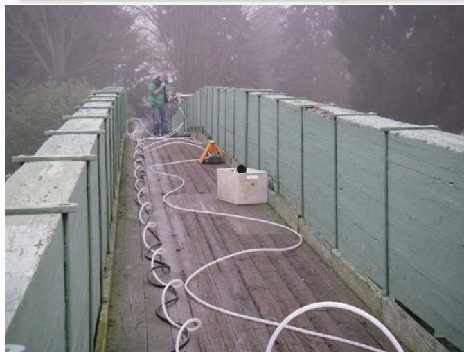
Figure B-3. Top - bridge boards used to lower and maintain position of pump. Middle - deploying a second pump into central channel. Bottom - running Teflon-lined tubing that will convey pumped river water along the bridge deck to the centrifuge trailer and sieving stations.
