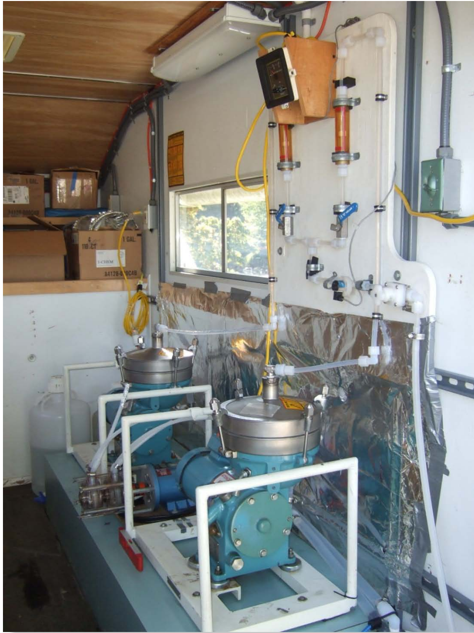
Figure B-4. Interior of trailer housing 2 Alpha Laval continuous flow-through centrifuges with influent flow controls.
