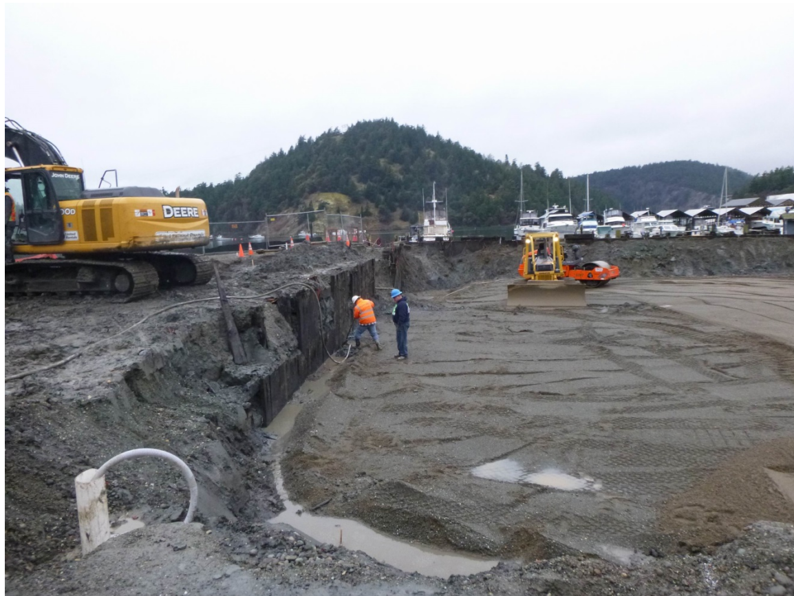
Figure 3: Overview of east side exposed southwest section of the bulkhead (view to northwest).
