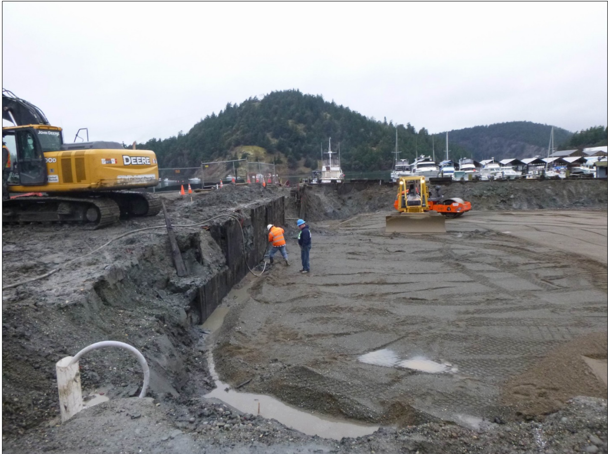
Figure 4-3 Overview of the southwestern extent of the bulkhead, view north. Goose rock can be seen in the background.
