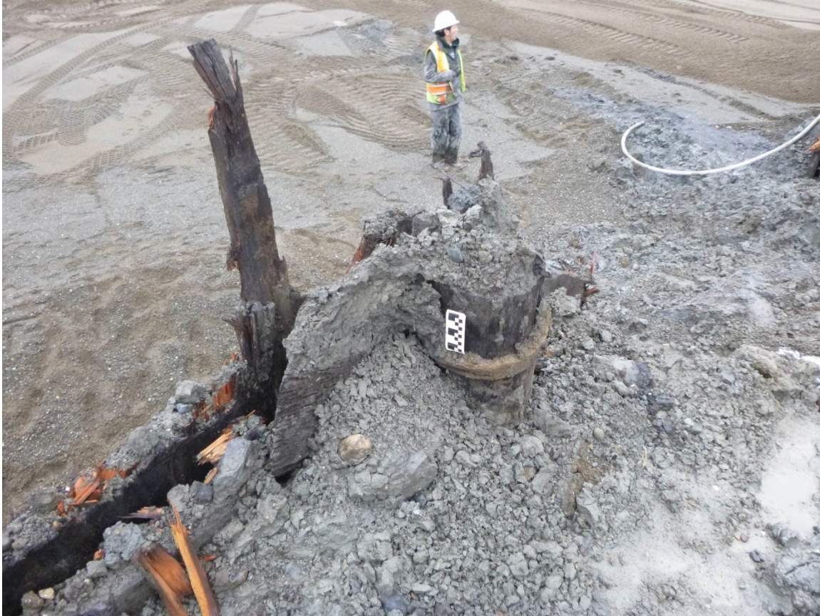
Figure 7: Overview of upper portion of a cable-wound support pile, showing diameter and size of cable (view to southeast).
