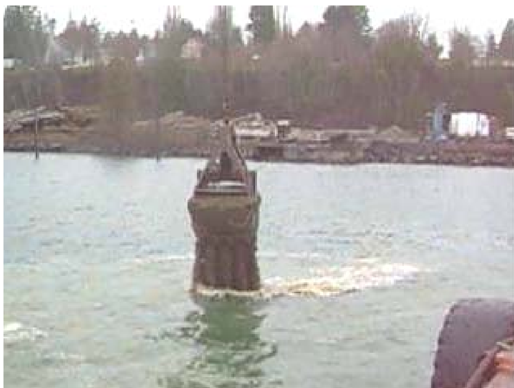
Photograph 21 - Sand cover placement with bucket above water to attain thin placement thickness. Note trail of air bubbles.
