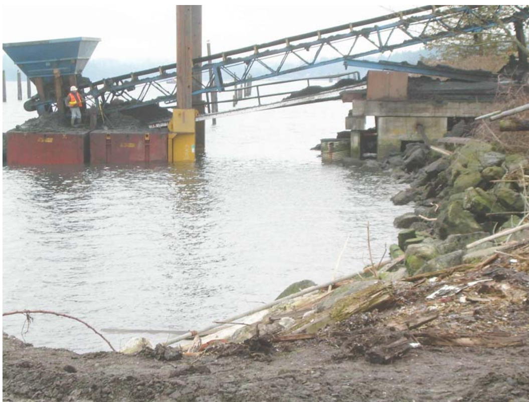
Photograph 13 - Offloading setup after planking installed between flexi-float (left) and upland structure (right) to catch sediment spilling off of conveyor.
