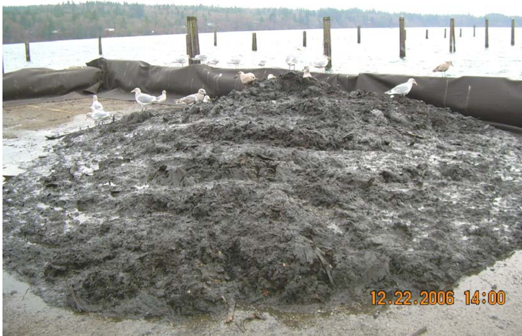
Photograph 6 - Wet dredge sediment excavated during test dredge (12/22/06). Sediment is predominantly the heterogeneous, dark (sandy) sediment/woodwaste-type dredged material.
