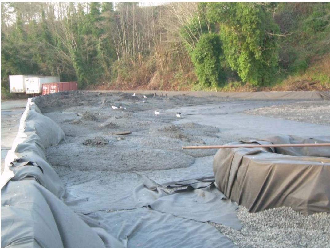
Photograph 16 - South end of sparging basin with wet silty dredge sediment at beginning of project. Note outfall inlet ecology blocks and geotextile at right in foreground.
