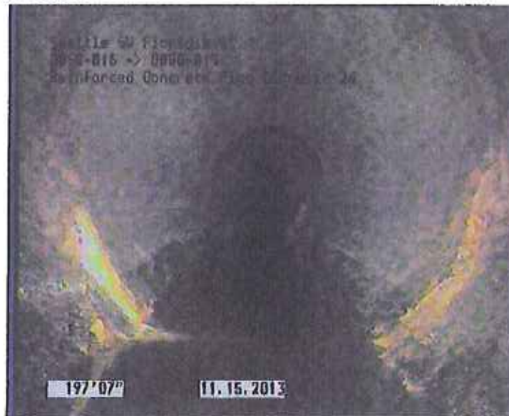
Photo: D050-016_D050-015_SW Florida St_15112013_091234_A.JPG, VCR No.: URS 197.55FT, Deposits Attached Encrustation, 5 %of cross sectional area, from 03 to 05 o'clock, , within 8 inches of joint: YES
