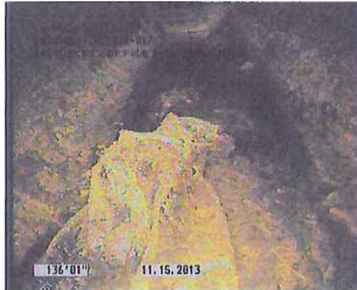
Photo: D050-017_D050-016_SW Florida St_15112013_083248_A.JPG, VCR No.: URS 136FT, Deposits Settled Other, 5 %of cross sectional area, from 08 to 07 o'clock, , within 8 inches of joint: YES / Unknown
