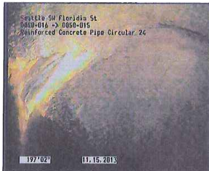
Photo: D050-016_D050-015_SW Florida St_15112013_091045_A.JPG, VCR No.: URS 197.2FT, Infiltration Runner, from 07 to 08 o'clock, within 8 inches of joint: YES
