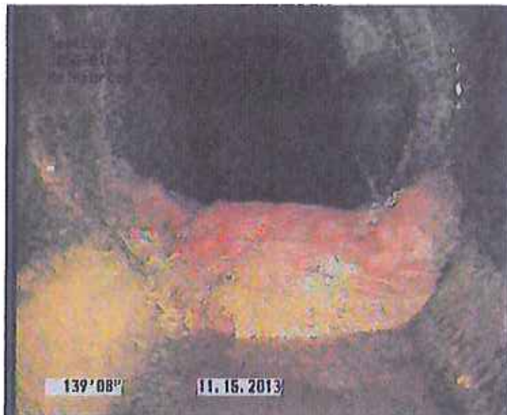
Photo: D050-017_D050-016_SW Florida St_15112013_083630_A.JPG, VCR No.: URS 142.85FT, Obstacles Other, 25 %of cross sectional area, from 04 to 08 o'clock / Absorbent Boom
