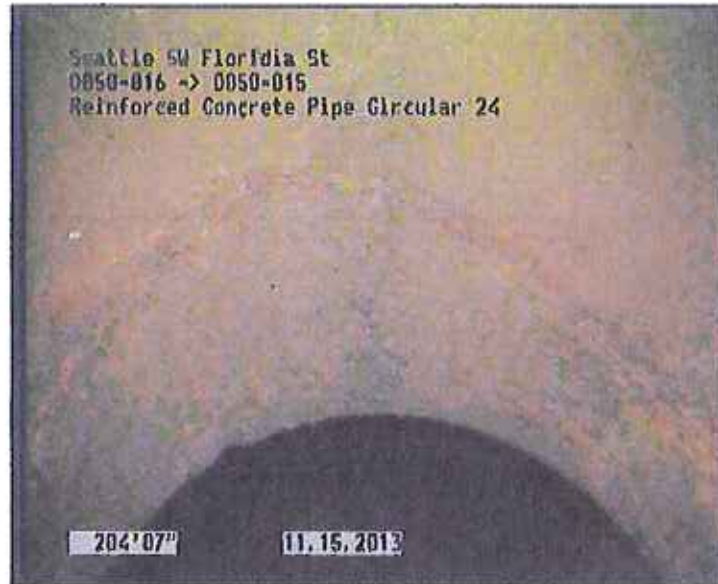
Photo: D050-016_D050-015_SW Florida St_15112013_091411_A.JPG, VCR No.: URS 204.6FT, Crack Circumferential, 10", from 09 to 03 o'clock, within 8 inches of joint: YES
