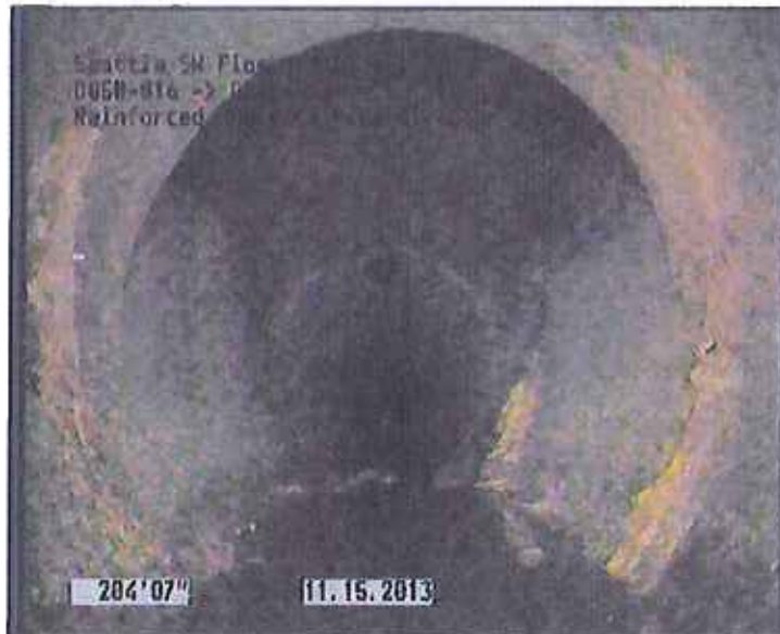
Photo: D050-016_D050-015_SW Florida St_15112013_091446_A.JPG, VCR No.: URS 204.6FT, Deposits Attached Encrustation, 5 %of cross sectional area, from 03 to 09 o'clock, , within 8 inches of joint: YES
