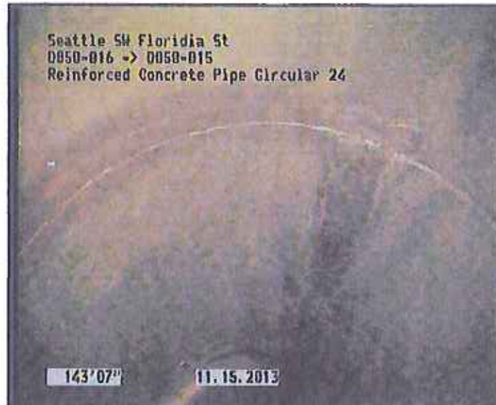
Photo: D050-016_D050-015_SW Florida St_15112013_085950_A.JPG, VCR No.: URS 143.6FT, Crack Circumferential, 6", from 09 to 12 o'clock, within 8 inches of joint: YES
