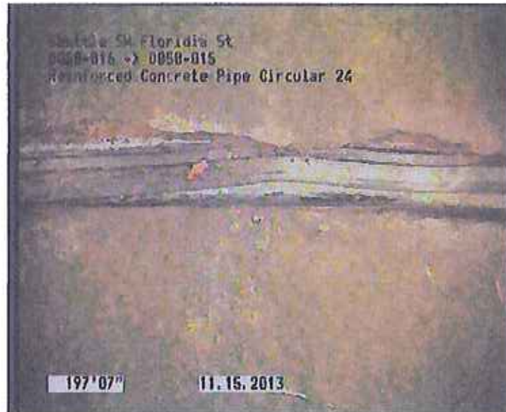
Photo: D050-016_D050-015_SW Florida St_15112013_091153_A.JPG, VCR No.: URS 197.55FT, Intruding Sealing Ring, 20 %of cross sectional area, from 09 to 03 o'clock
