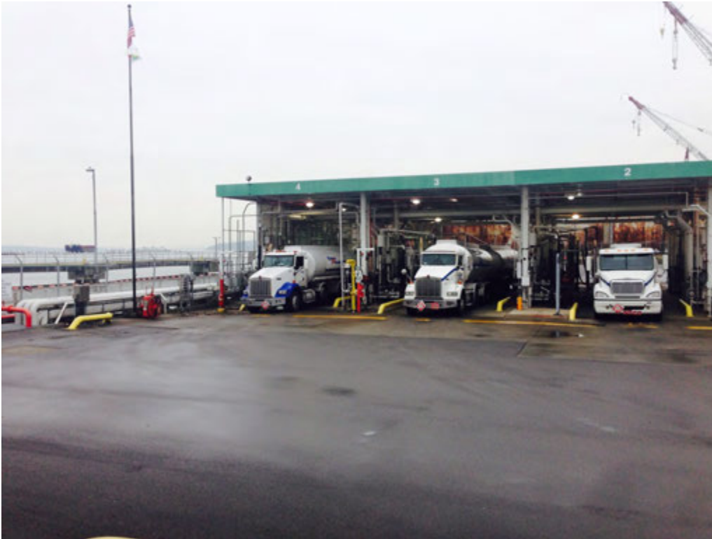
Photo 1. BP Terminal Harbor Island illustrating one petroleum fuels loading rack looking northwest.
