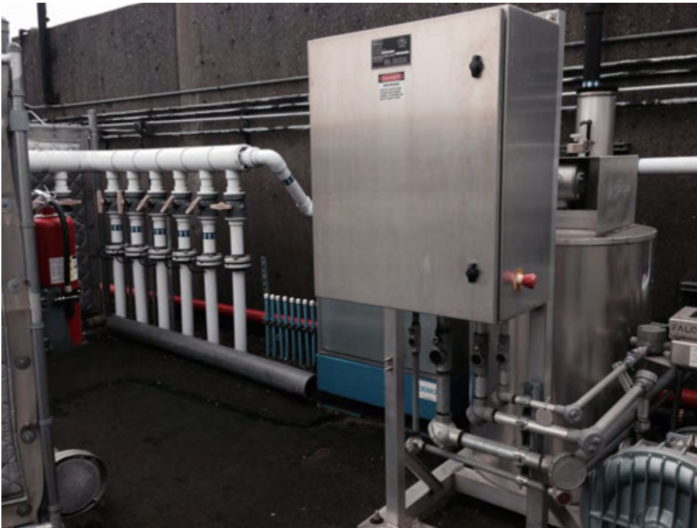
Photo7. BP Terminal Soil Vapor Extraction Remediation System equipment is shown with pumping station, vapor removal and stripping system and six individual well piping with control valves. This system is removing petroleum vapors from soil and groundwater for subsurface cleanup action.
