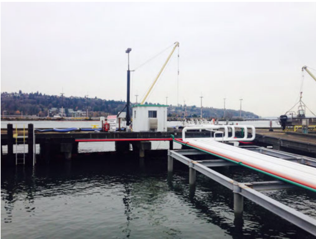
Photo 4. BP Terminal continuation of photo 2 showing on-loading and off-loading petroleum fuels piping and dock at West Waterway looking westward in distance is the north edge of West Seattle.
