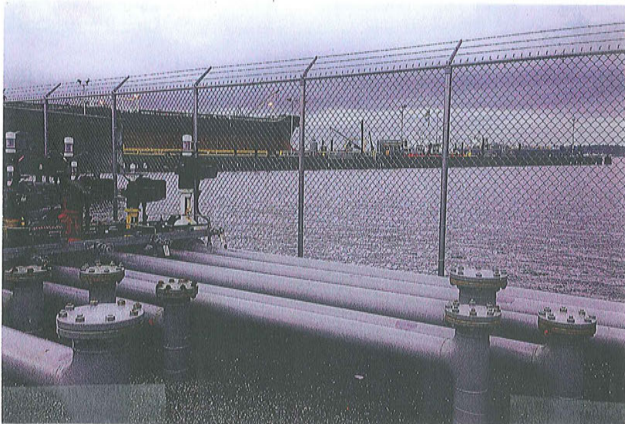
Photo 3. Shell Shoreline Manifold Area looking northwest to Port of Seattle.
