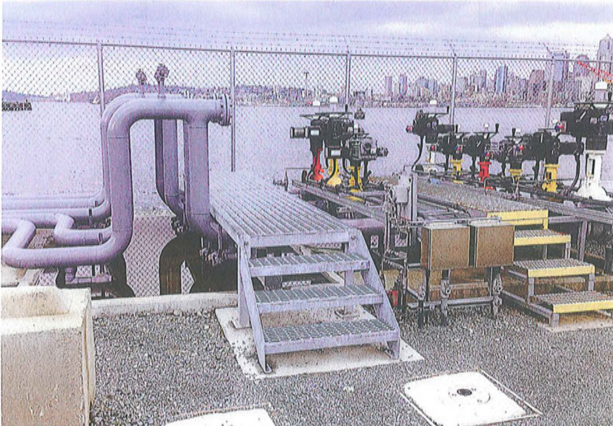
Photo 2. Shell Harbor Island Terminal Shoreline Manifold Area looking northeast across Elliott Bay to City of Seattle in background.
