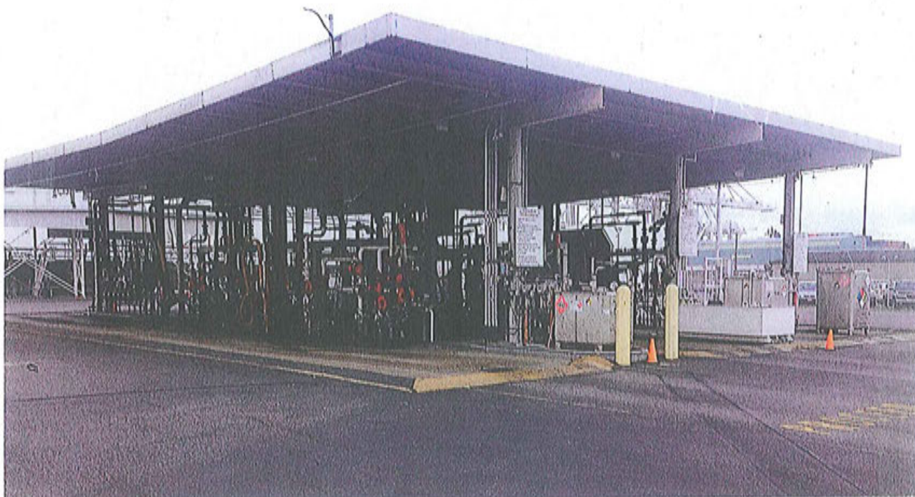
Photo 1. KMLT illustrating a petroleum fuels loading rack.
