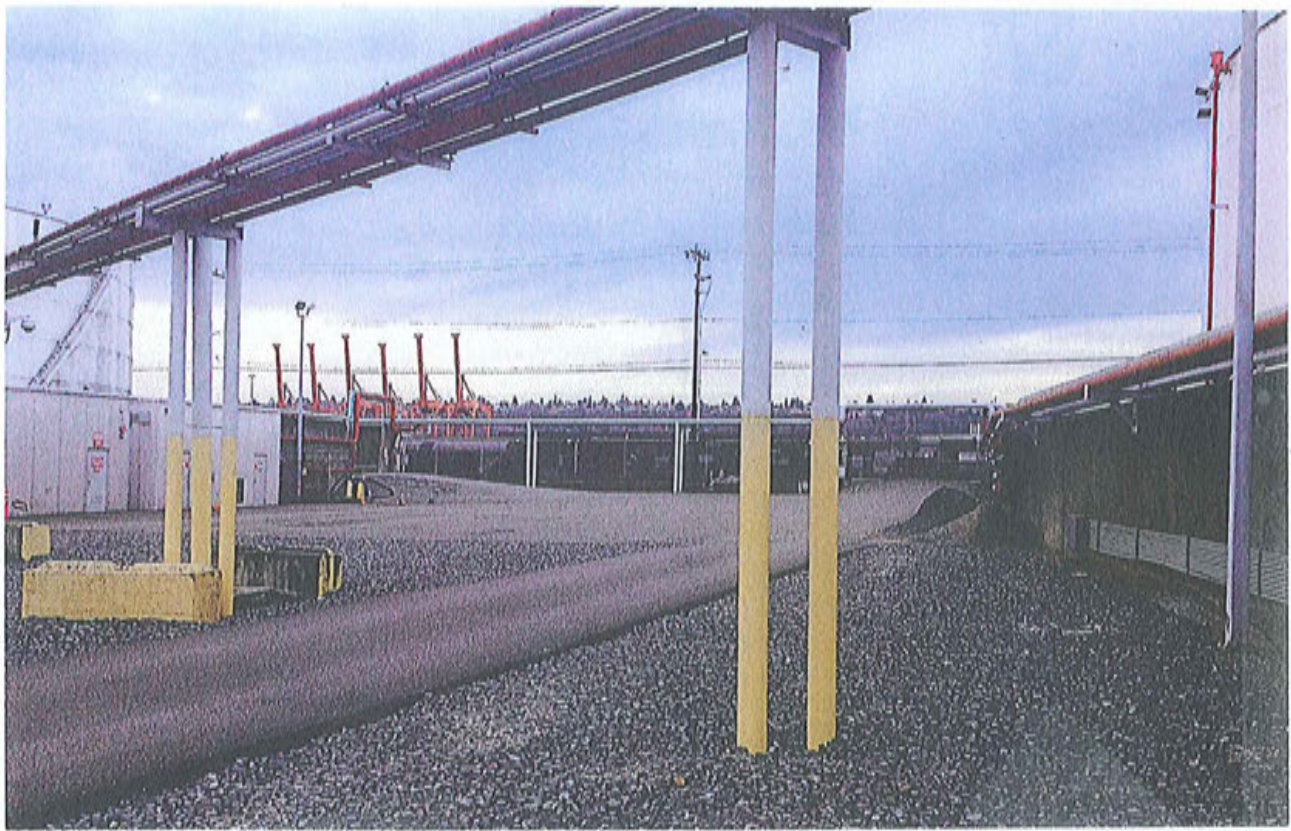
Photo 5. Overhead supply piping between KMLT yards showing impermeable (paved) and permeable (gravel) surfaces and current site conditions.
