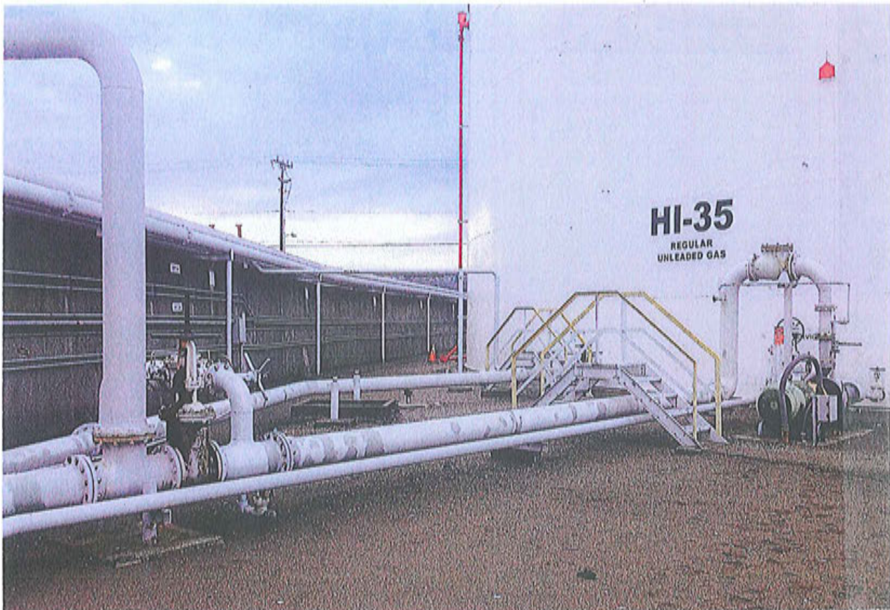
Photo 4. KMLT Above ground petroleum Storage Tank No 35 at E Yard with supply piping and valves.
