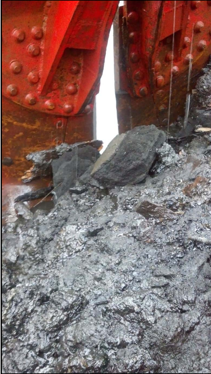
Photograph 12 – Compacted sandblast grit in dredge spoils (January 27, 2014).
