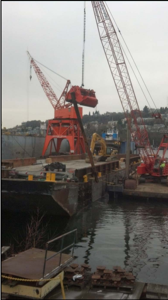
Photograph 16 – Example of timber pile recovered during dredging operations (December 5, 2013).
