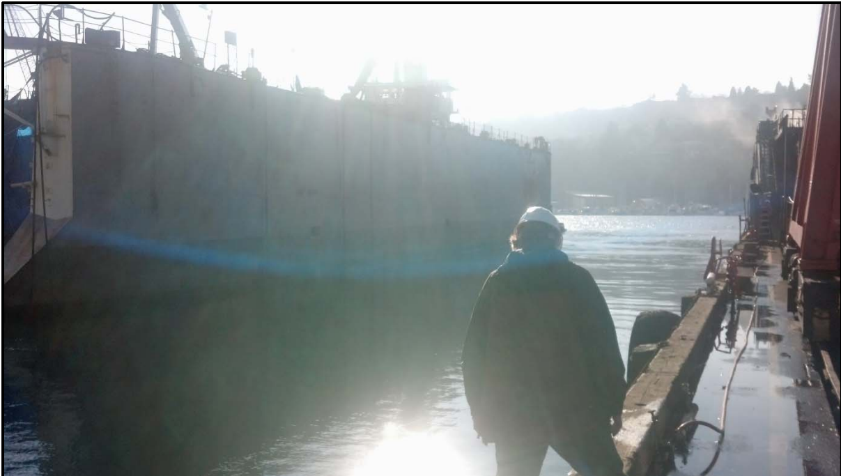
Photograph 21 – Northlake Shipyard relocating Dry Dock 9 to allow dredging operations to begin on the east side of the pier (January 23, 2014).
