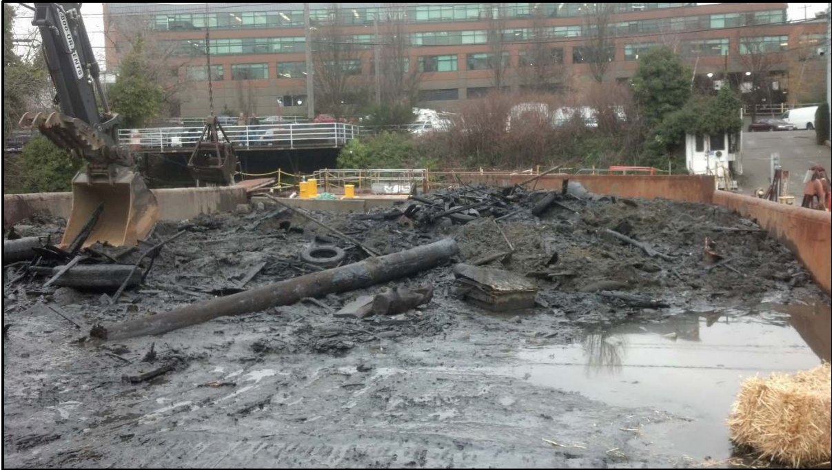
Photograph 10 – Dredge spoils and debris recovered from Waterway 21 (December 9, 2013).
