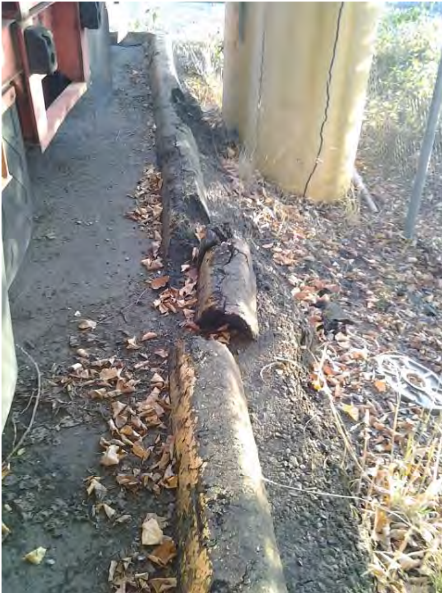
Photograph 5 – Northern curb damage.
