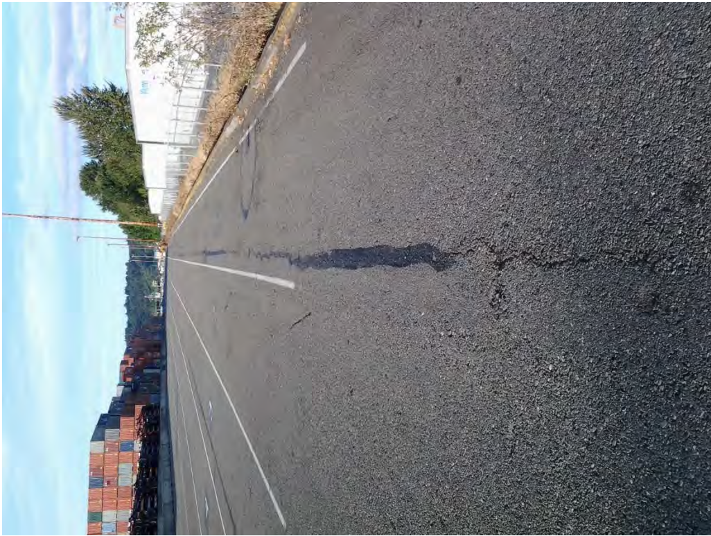
Photograph 1 – Pavement crack and deteriorating seal. (← Up)
