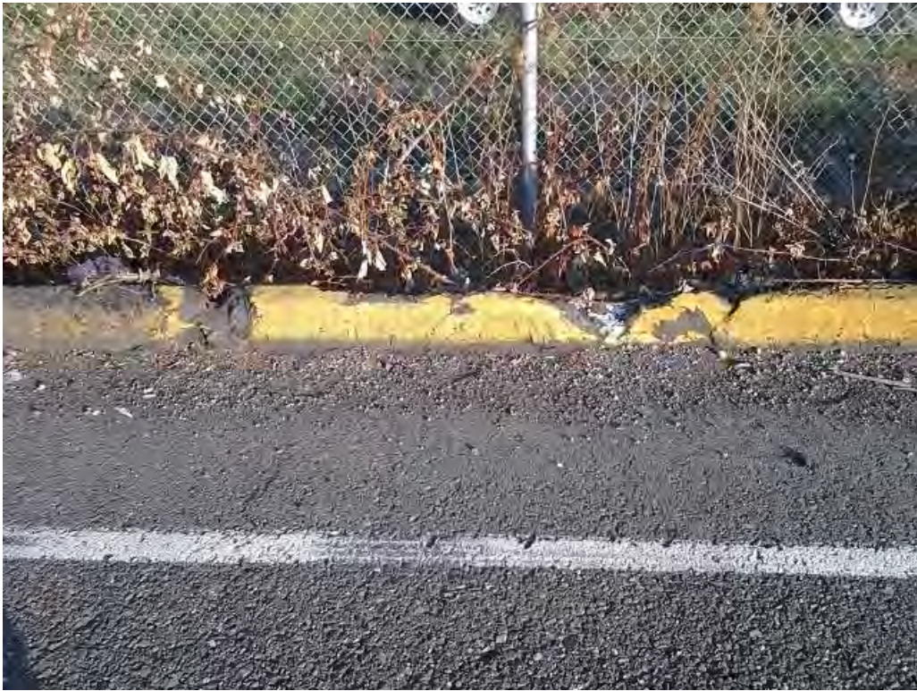
Photograph 3 – Southern curb damage.
