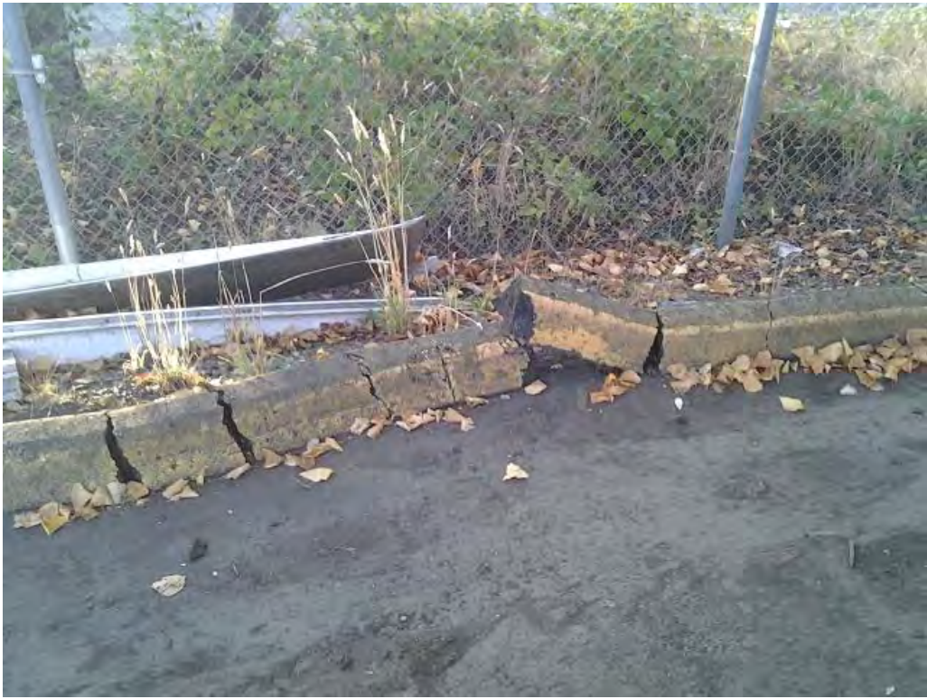
Photograph 4 – Northern curb damage.
