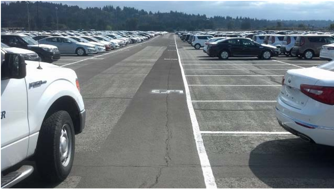
Photograph 3 – Observed cracks in cap.
