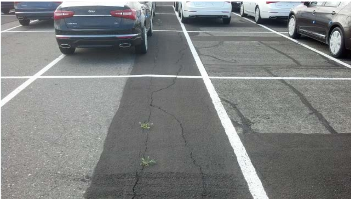
Photograph 2 – Observed cracks in cap.
