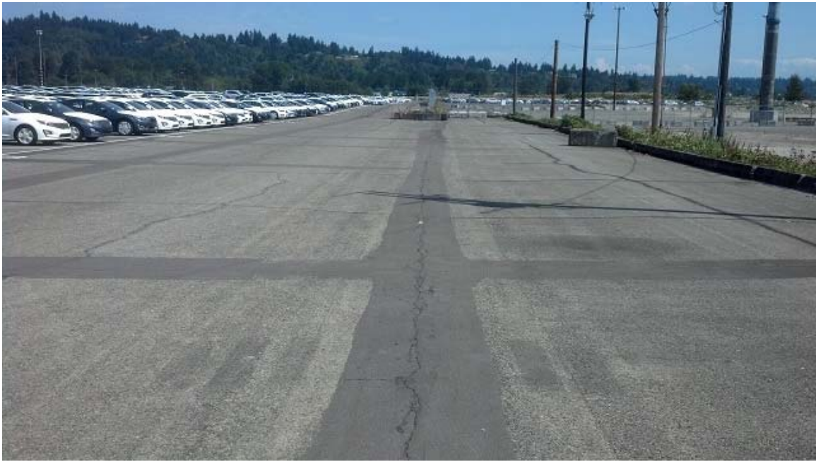
Photograph 4 – Observed cracks in cap.
