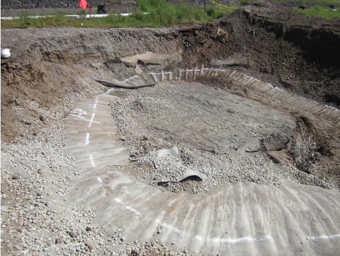
2014, May 13. East sinkhole.
