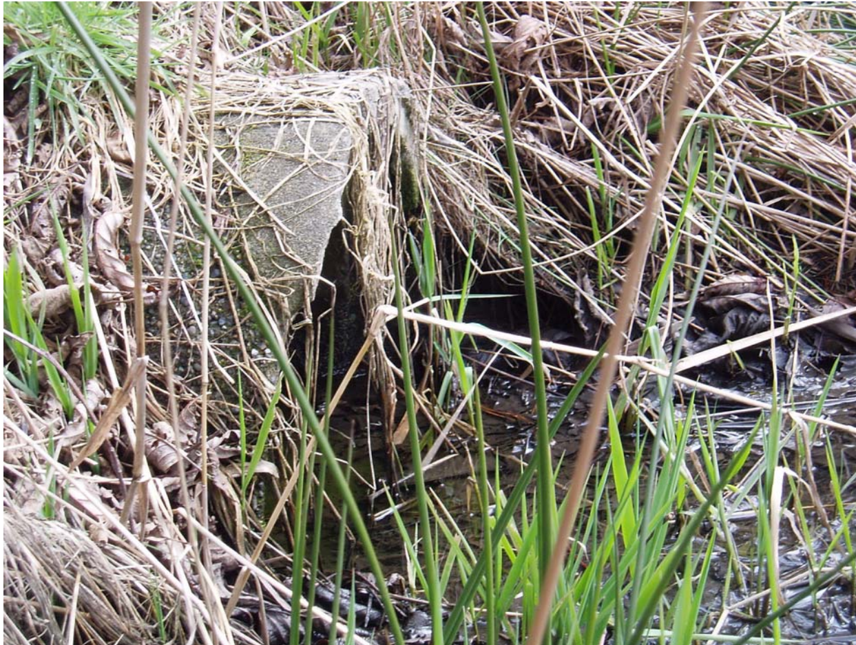
Photograph 5: No discharge was observed from the partially submerged concrete outfall.
