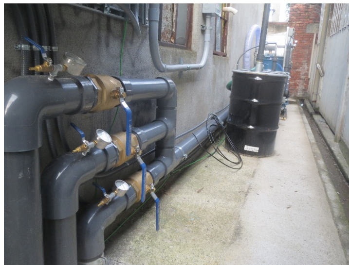
Photograph 2 – Manifold pipes, control valves, and vacuum gauges and sample ports for glacial till wells (VE-1/VE-2) on left, advance outwash wells (VE-3/VE-4) in middle, and SVE trench (VE-H) on right.
