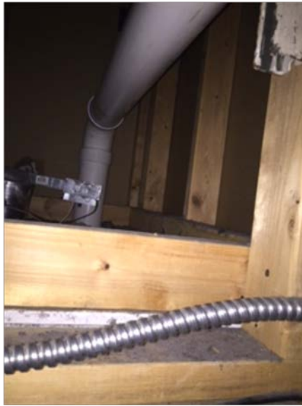
Photograph 5 – VE-SS lateral pipe that connects to SVE system. This may be extended through ceiling and connected to radon fan after sufficient SVE treatment.
