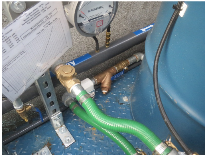
Photograph 12 – Pitot tube flow meter on effluent line from the vapor liquid separator.
