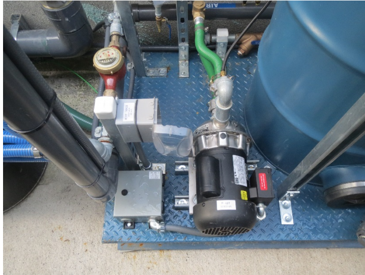
Photograph 13 – Water transfer pump for the vapor-liquid separator.
