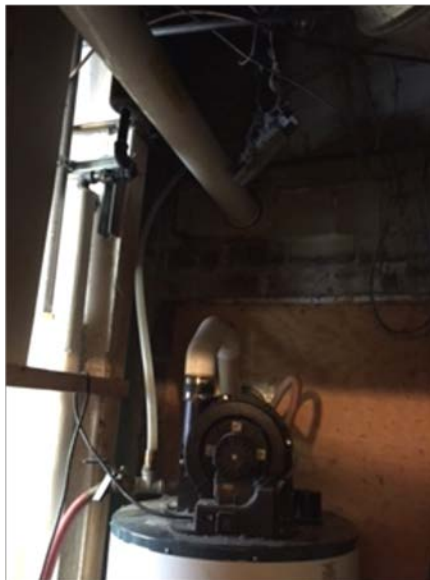
Photograph 6 – Lateral extension of VE-SS pipe through north sidewall of Morrell's Dry Cleaners.
