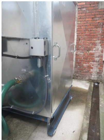
Photograph 10 – Sound proof enclosure that contains the 2-HP regenerative blower.
