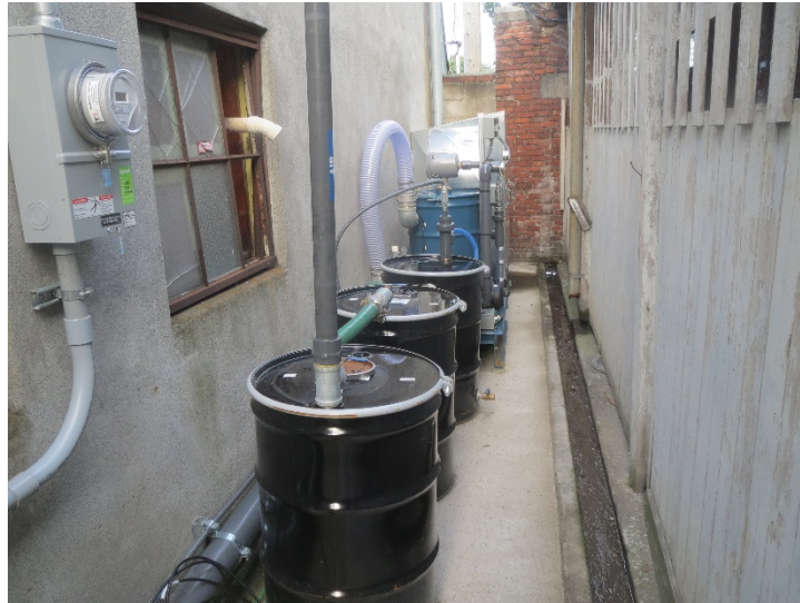
Photograph 9 – SVE system, including 2 GAC drums in foreground, water collection drum (3 rd drum), vapor liquid separator (blue drum), and blower housing in back.
