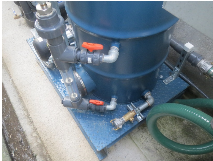
Photograph 14 – Site gauge on the vapor liquid separator.
