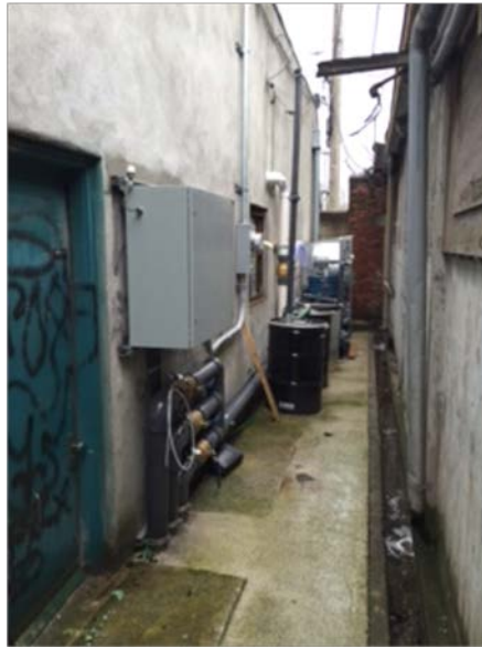
Photograph 1 – Soil vapor extraction (SVE) system installed in the 5-foot-wide alley on the north side of Morrell’s Dry Cleaners.
