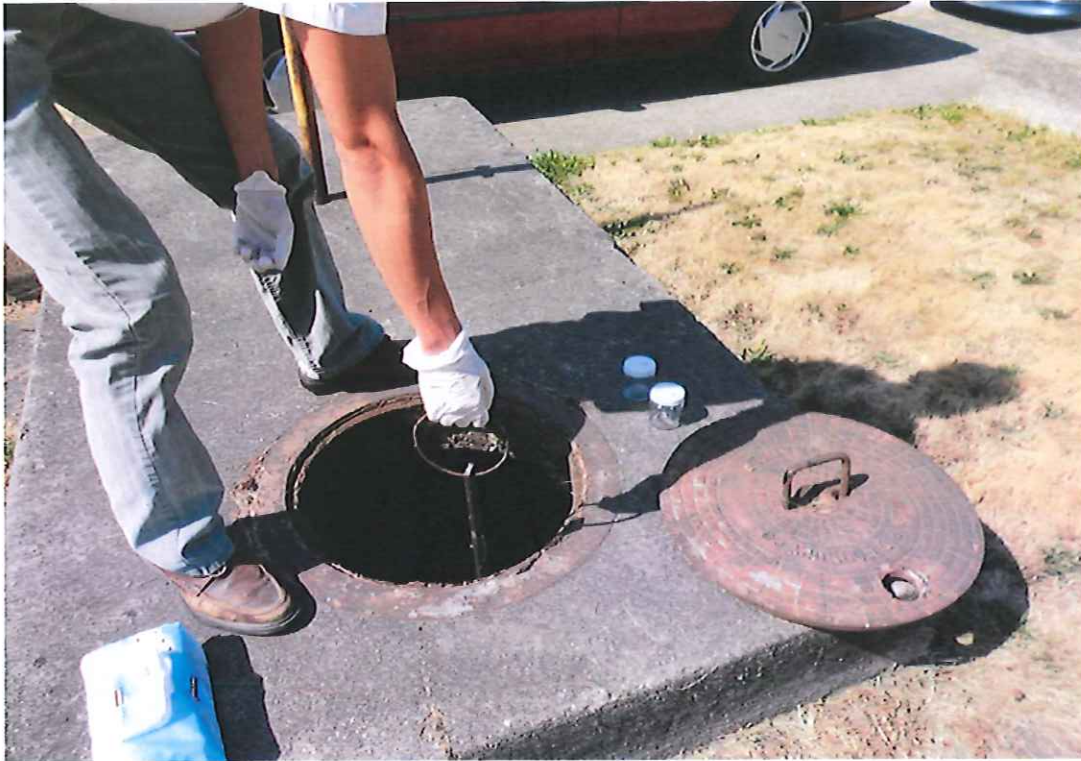
Photograph 3: View of UST 3 fill port with dip stick on the east side of the tank.
