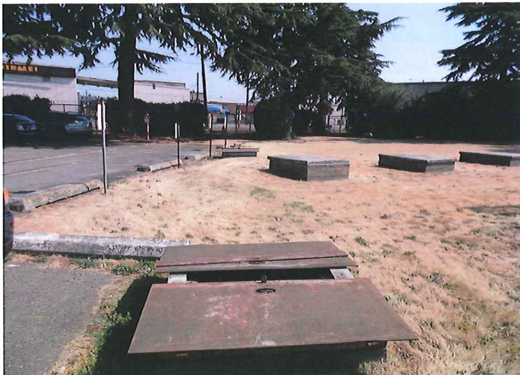
Photograph 4: View of the USTs location from the west, in foreground is a fuel pump vault and the fill port vault are seen in the background.
