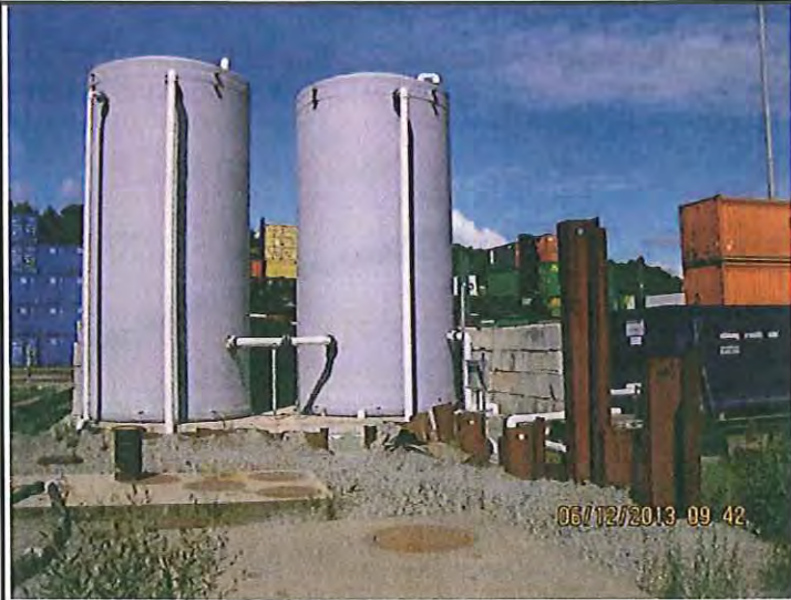
#5. DESCRIPTION: These tanks collect and store stormwater that feeds the treatment system.
