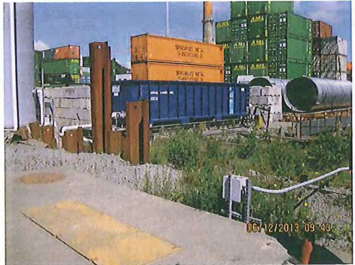
#4. DESCRIPTION: The StormwaterRx system treats all stormwater from Zones A and D which comprises approximately 70 percent of the facility.
