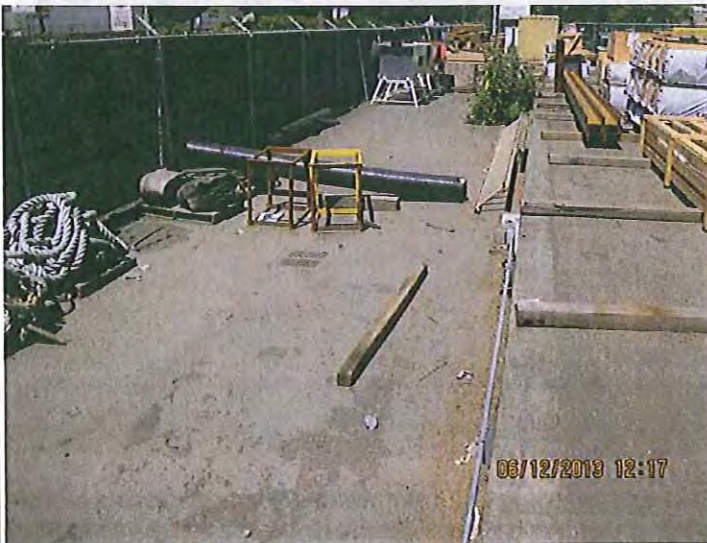
#15. DESCRIPTION: The SWPPP indicates that the storm drains in this area can be directed to the sanitary sewer or to Zone "B", which flows to Outfall # DP-1. SPU later determined that there are no sanitary sewer connections in this area.
