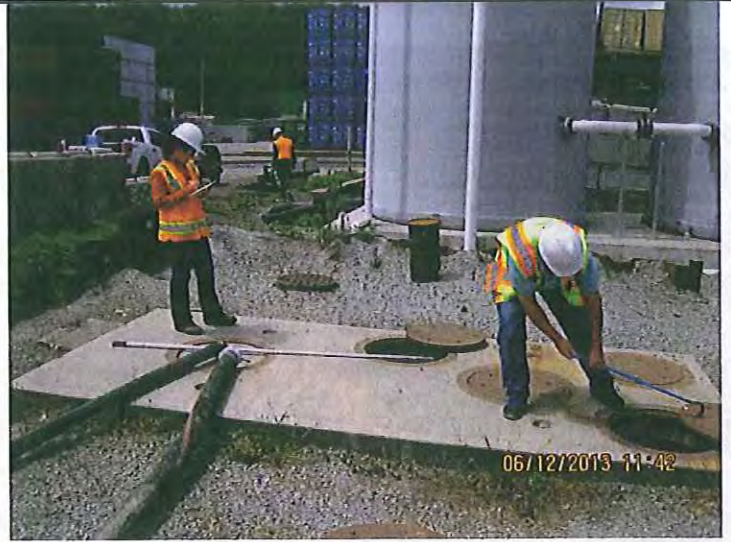
#6. DESCRIPTION: The stormwater plumbing in this area is complicated. The facility must include a more detailed diagram of the Contech Vortechs and Storm Filter vaults, tanks, pumps and piping in this area.
