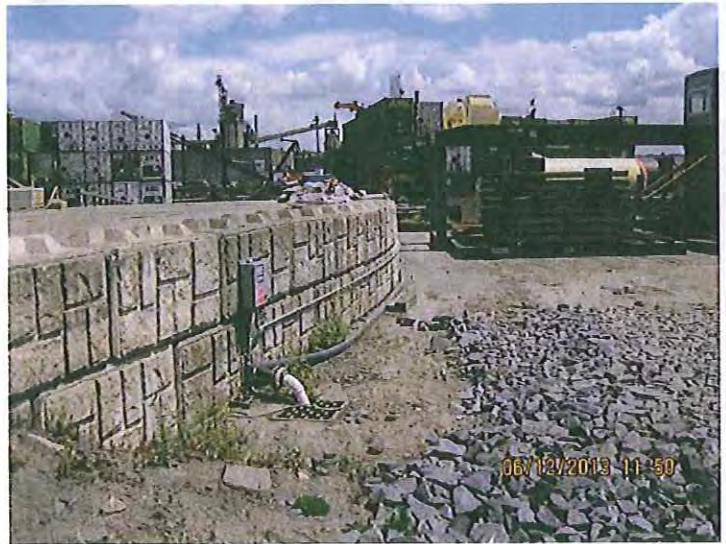
#8. DESCRIPTION: The area at the southeast corner of the facility is Zone "D". This could use improved source control measures to stabilize the bare soils.
