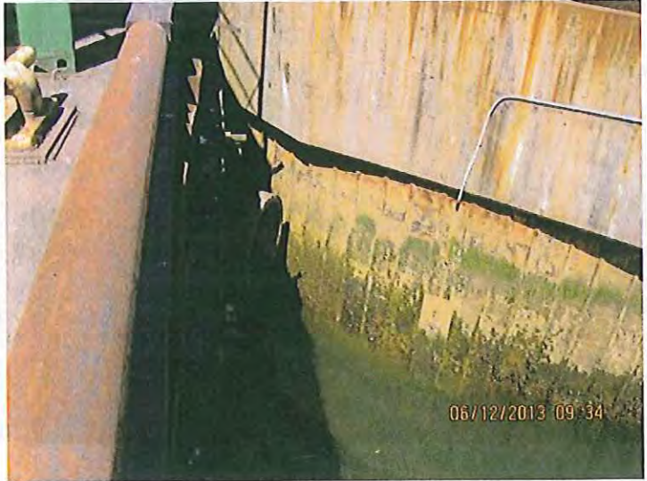
#2. DESCRIPTION: Approximately 20 percent of the site drains to the sand filters the northern edge of the property. Outfall # DP-1, seen above, rarely discharges.
