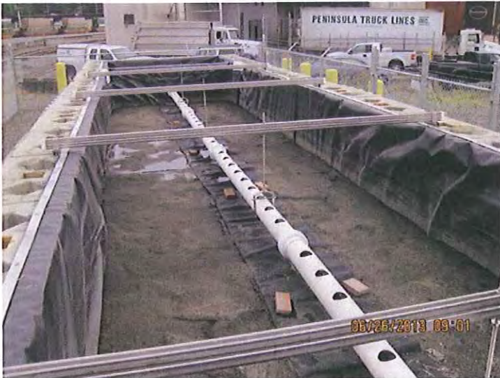
#1. DESCRIPTION: Union Pacific Railroad triggered Level 3 corrective actions for turbidity. They are in the final stages of completing the construction of Level 3 StormwaterRx sand filter treatment systems.
