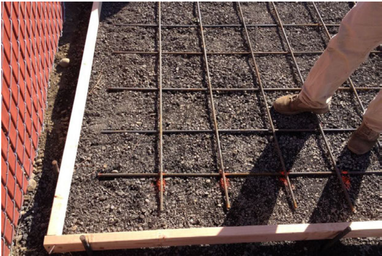
Photograph 8 – GTS concrete foundation form work and reinforced rebar grid. Rebar is spaced 12 inches apart.
