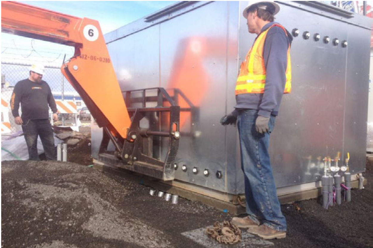
Photograph 11 – Installation of the GTS building on the concrete slab. Note four groundwater extraction pipes surfacing near the center of the building, four groundwater injection pipes surfacing near the right of the building, and an electrical pull box shown in the foreground. Photograph taken facing northeast.
