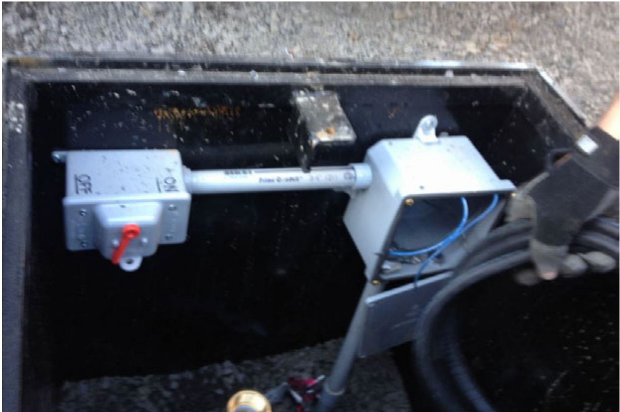
Photograph 27 – Typical electrical boxes installed in extraction well vaults. Manual pump on/off switch provided on the left with electrical connection/pull box on the right.
