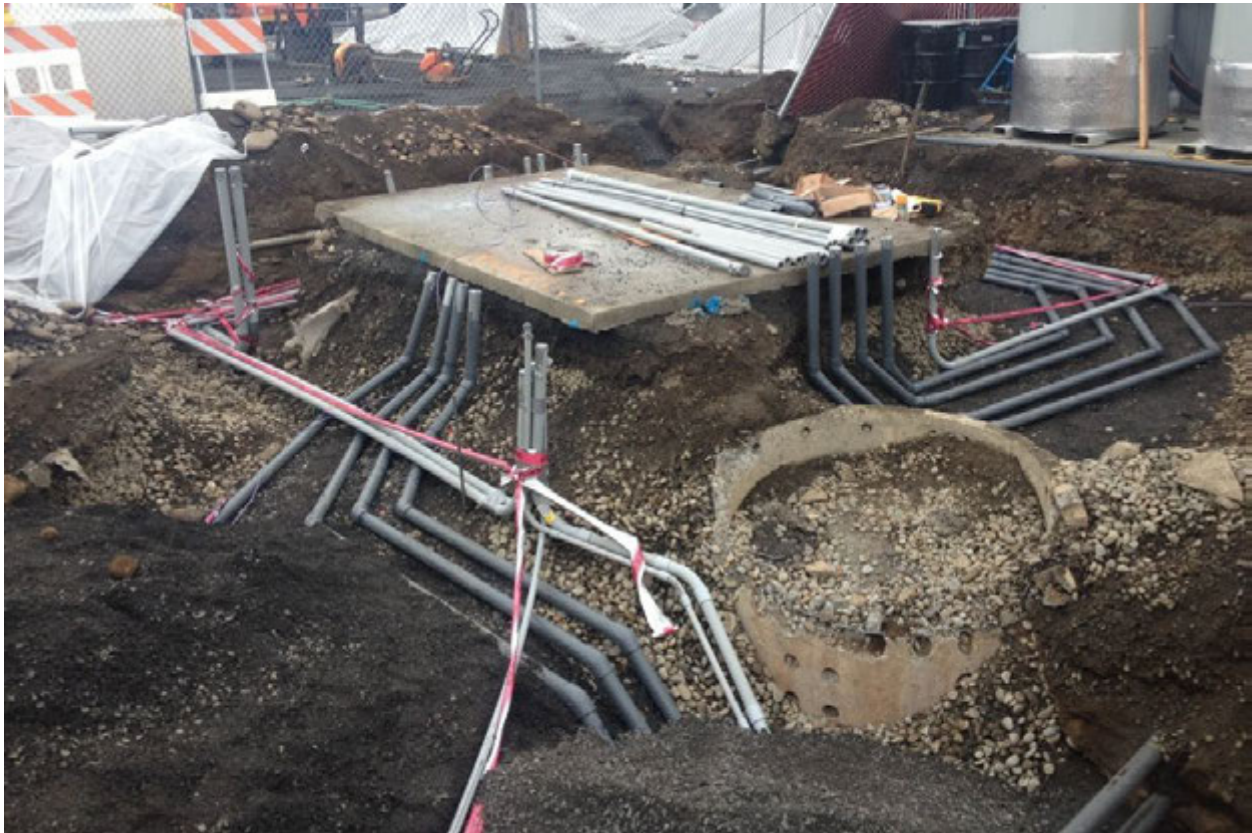
Photograph 21 – Photograph shows GTS building foundation slab with excavation on all sides for pipe installation. Extraction well pipes are in the foreground on the left. Extraction well conduit crosses over the conveyance pipe and wraps around the slab. Injection well pipe wraps around the slab on the right with electrical conduit for batch tank accessories currently sitting on the pipe. The abandoned dry well is visible in the foreground. Photograph taken facing northeast.
