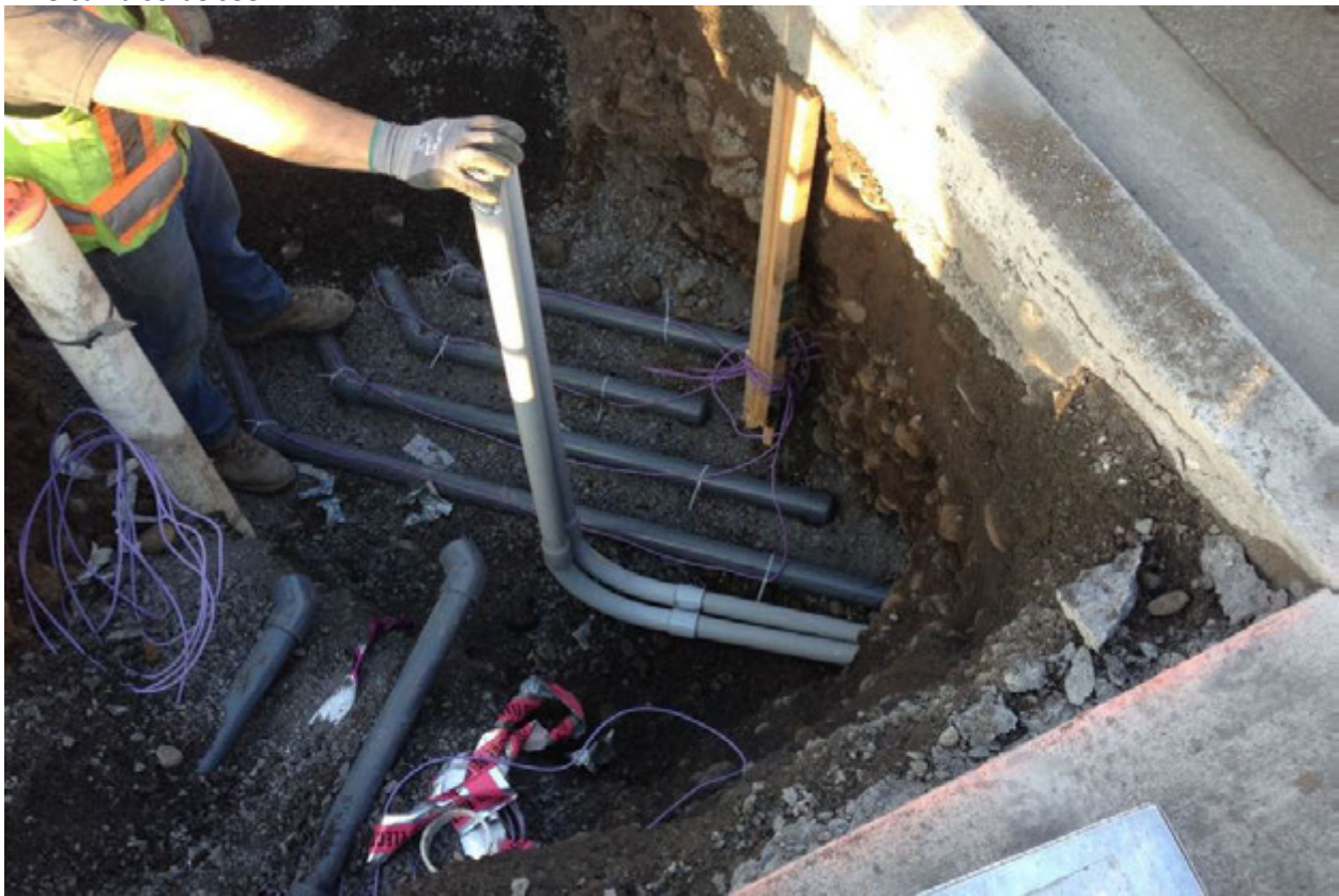
Photograph 20 – Photograph shows intersection of conveyance pipe and electrical conduit (employee is holding) at EXT-4 (white vertical pipe with orange cap). Four lower pipes on the right are capped in the photograph for future installation. Two pipes on the left are conveyance pipe for EXT- and EXT-3. South 3rd Ave. is on the right.
