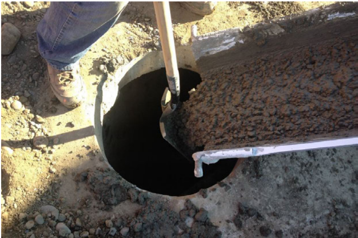
Photograph 30 – Photograph shows decommissioning of drywell on the Site by filling with leftover concrete after pouring GTS building foundation slab.
