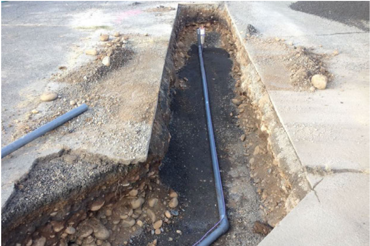
Photograph 17 – INJ-1 trench with conveyance pipe installed over compacted bedding material with tracer wire attached. Photograph taken facing west.
