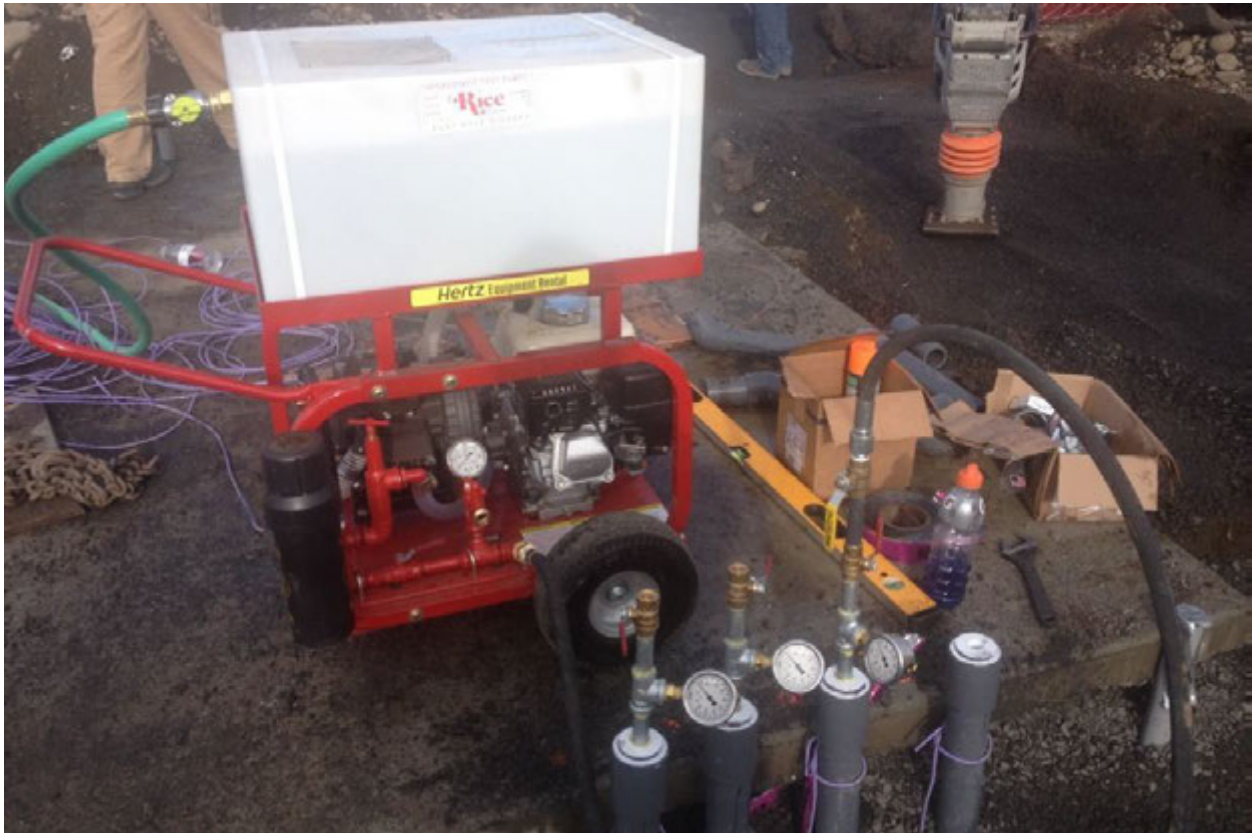
Photograph 25 – Hydrostatic pressure tester sitting on GTS foundation slab connected to injection well piping. Photograph taken facing north-northeast.
