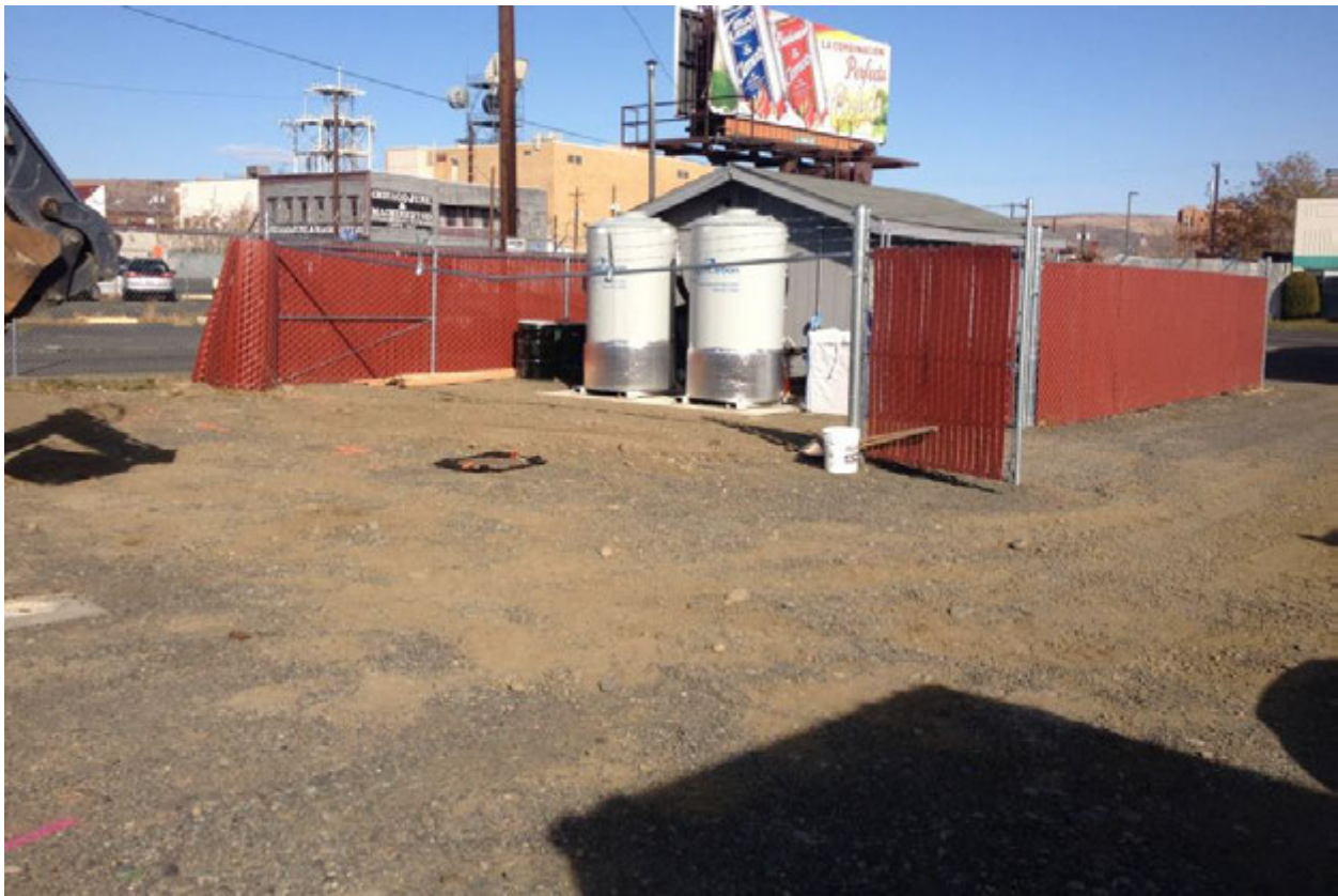
Photograph 4 – SVE System enclosure opened up during site preparation activities. GTS to be installed to west of SVE system and existing fence extended. Photograph taken facing northeast.
