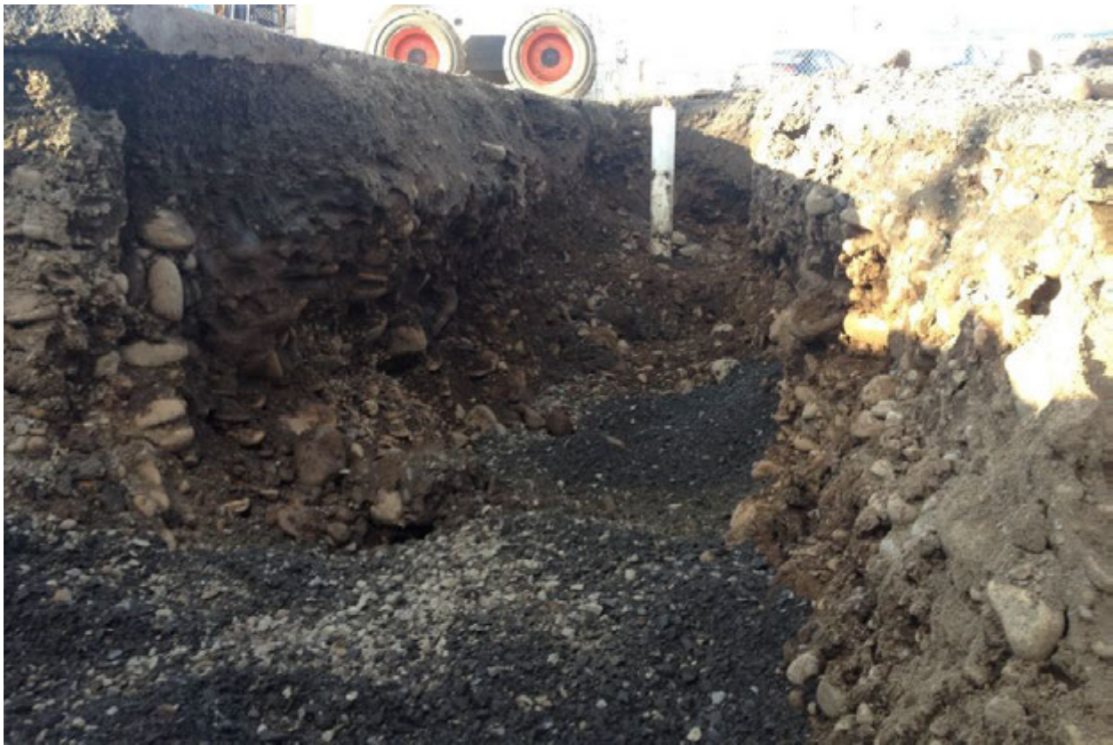
Photograph 14 – Trenching to INJ-1 (well casing visible) showing typical cave-in issues encountered within trenches. In this photograph the pipe bedding material was loosely placed when cave-in occurred. Photograph taken from within INJ-1 trench facing west.
