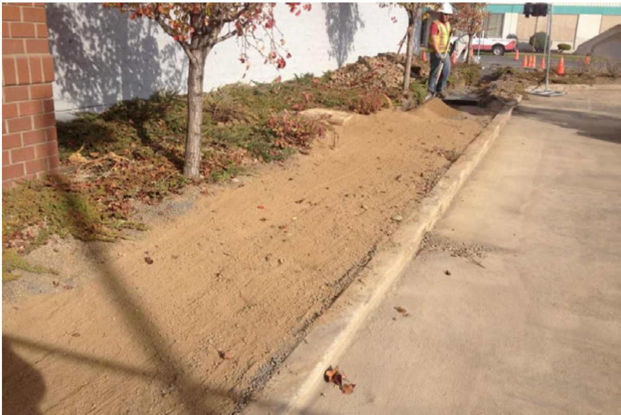
Photograph 24 – Extraction well EXT-2 and EXT-3 trench surface material within landscaped area of CWCMH facility property. Photograph taken facing east.
