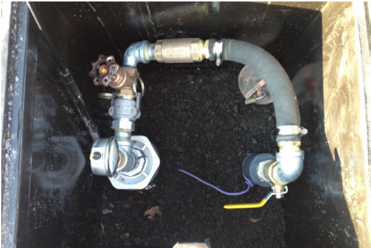
Photograph 26 – Typical injection well vault showing wellhead connections.
