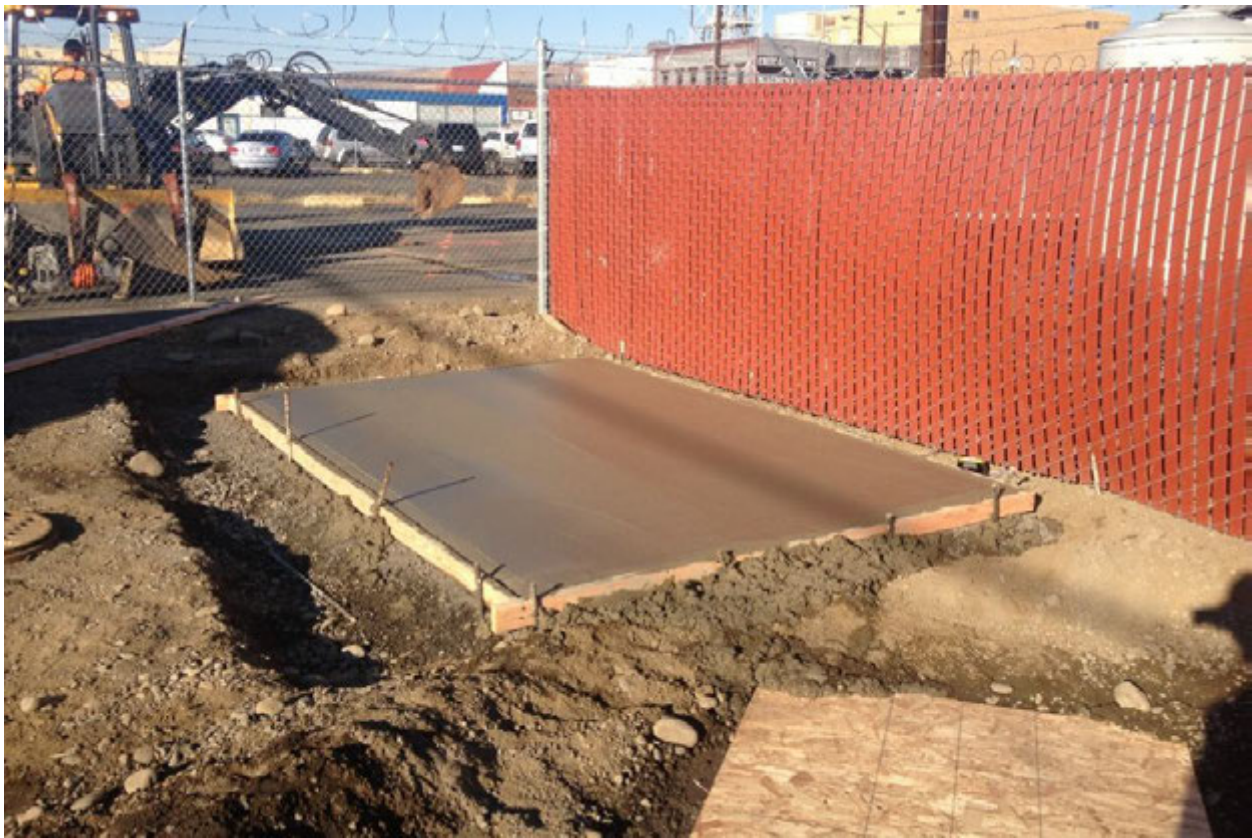
Photograph 10 – Concrete slab poured. Private asphalt parking lot shown in the background with SVE system fence to the right. Photograph taken facing northeast.
