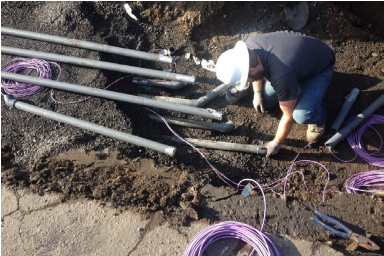
Photograph 19 – This photograph shows a second row of conveyance pipes placed over a lower row of installed pipe. Contractor is installing fittings on lower row in photograph. Purple coils of utility tracer wire can also be seen.
