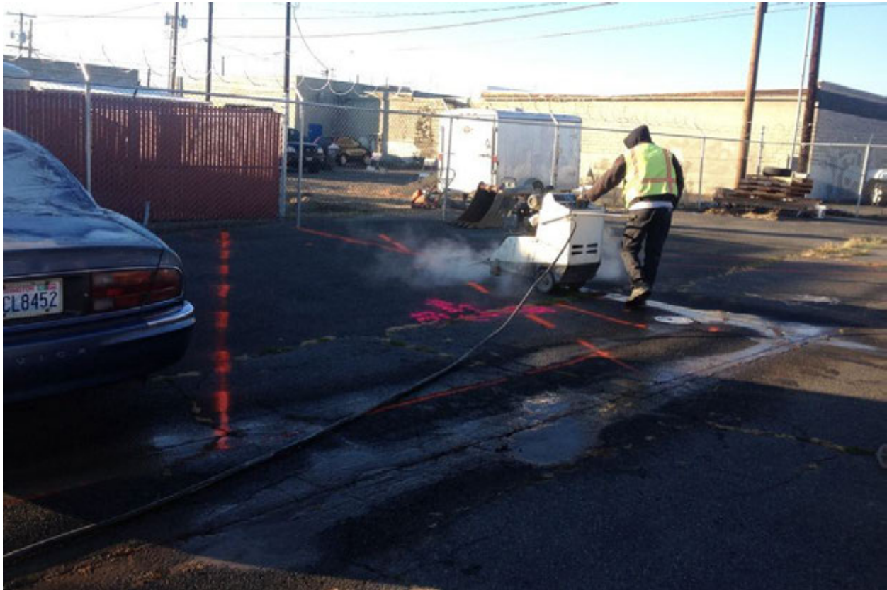
Photograph 13 – Concrete cutting on the private parking lot north of the Site. Injection well INJ-2 can be seen behind the employee. Photograph taken facing southwest.
