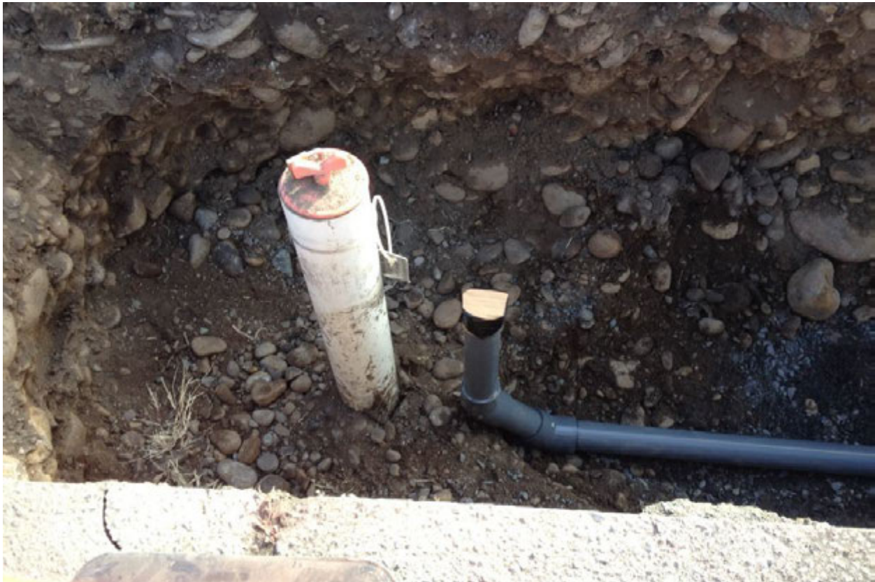
Photograph 15 – Typical well casing (white) with conveyance pipe (gray).
