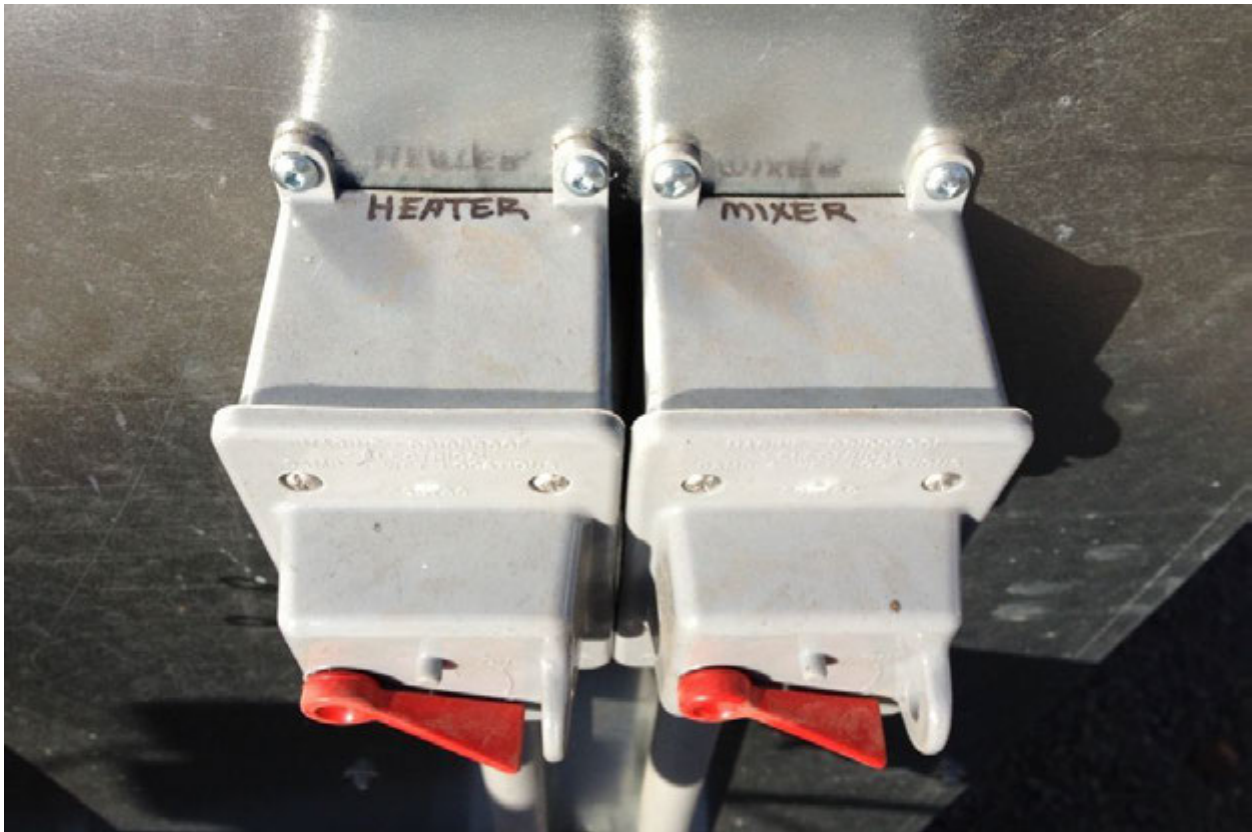
Photograph 12 – External switches installed on the GTS building to control batch tank mixer and heater.
