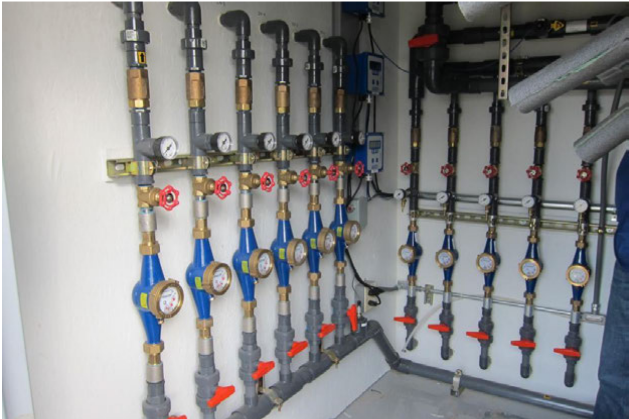
Photograph 7 – Inside of the GTS, photograph shows the injection well manifold on the left and a portion of the extraction well manifold on the right.
