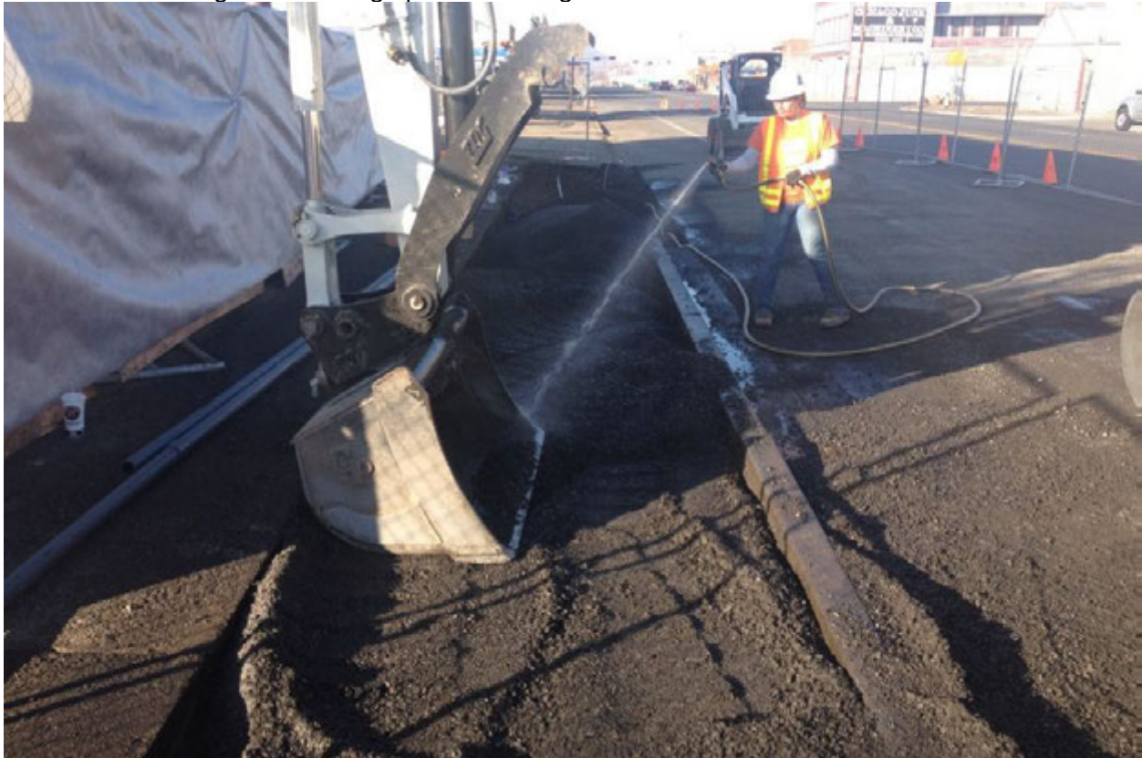
Photograph 22 – Wetting trench backfill while placing along S 3rd Ave. Photograph taken facing north.
