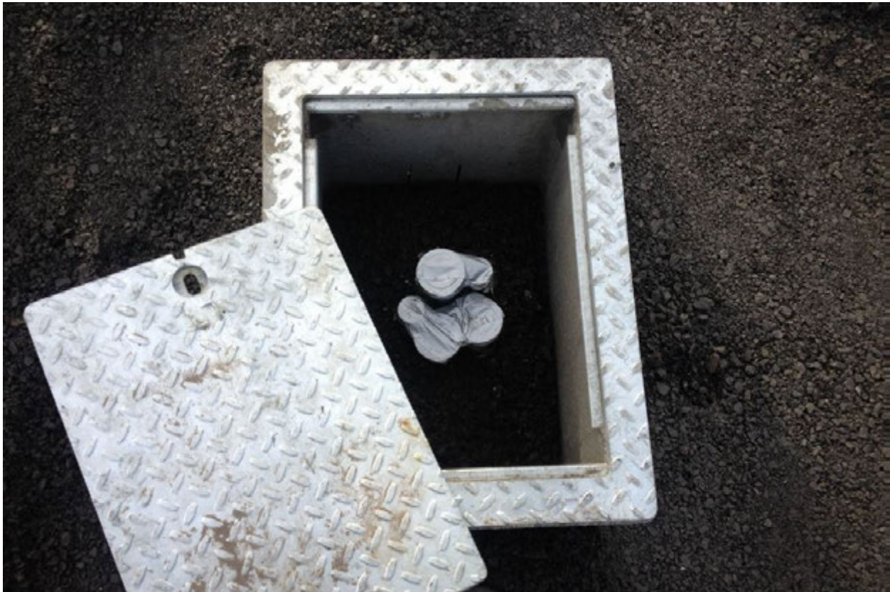
Photograph 29 – Typical electrical pull box vault.
