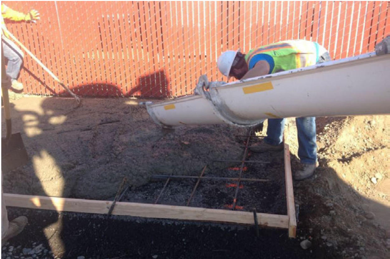
Photograph 9 – ERRG staff working concrete mixture and positioning rebar grid while pouring concrete foundation. Treatment compound fence shown in the background. Photograph taken facing east.
