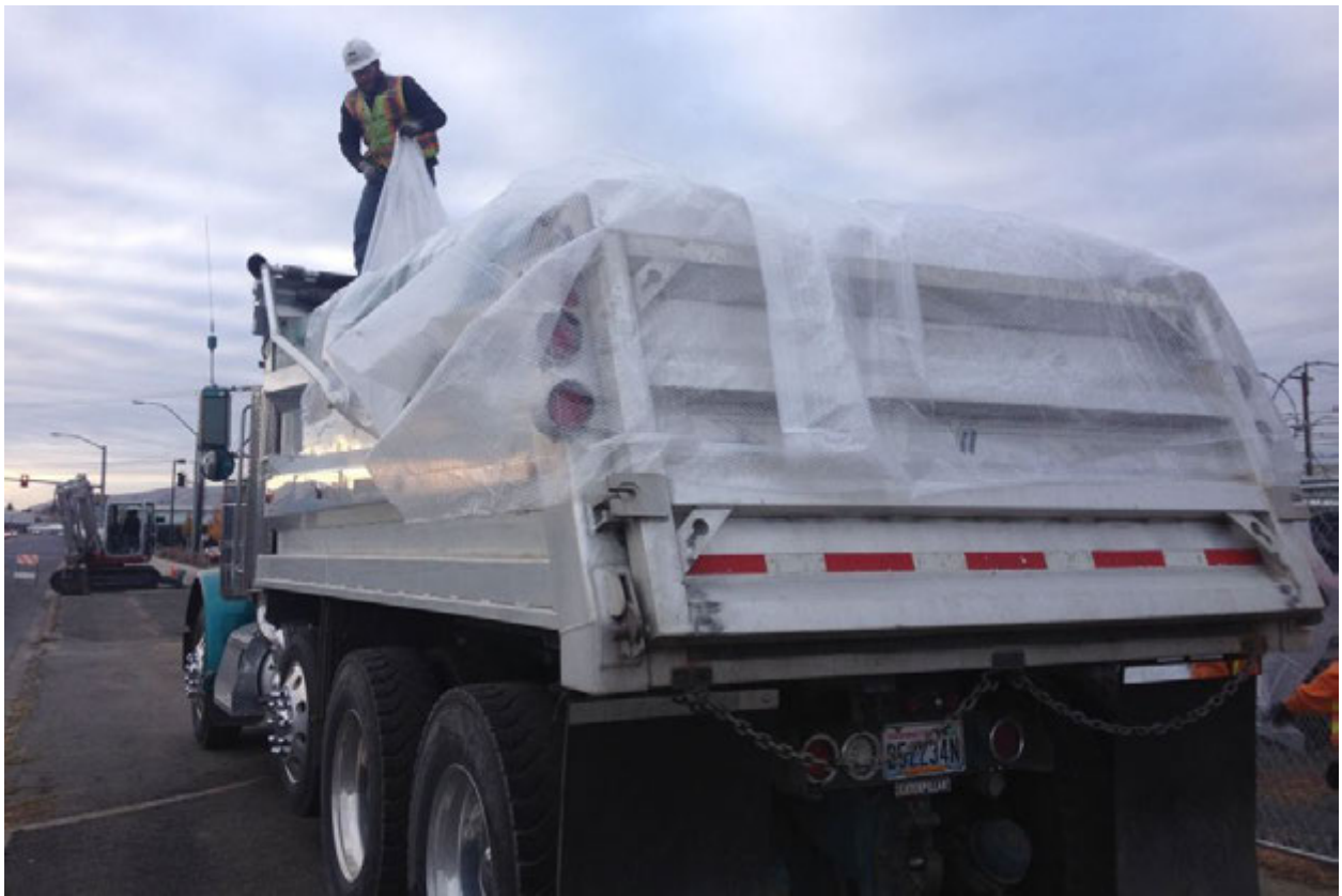
Photograph 32 – Truck bed liner being lined with plastic for impacted soil disposal. Photograph taken facing south.
