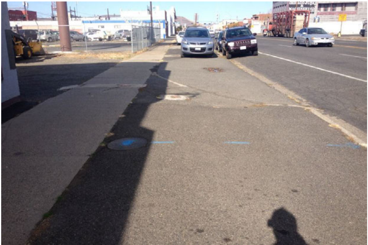
Photograph 2 – South 3rd Avenue sidewalk conditions prior to construction. Children’s daycare water service line marked in blue in foreground. Photograph taken facing north.
