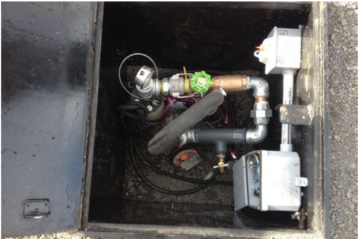
Photograph 28 – Typical extraction well vault showing wellhead connections and electrical components.
