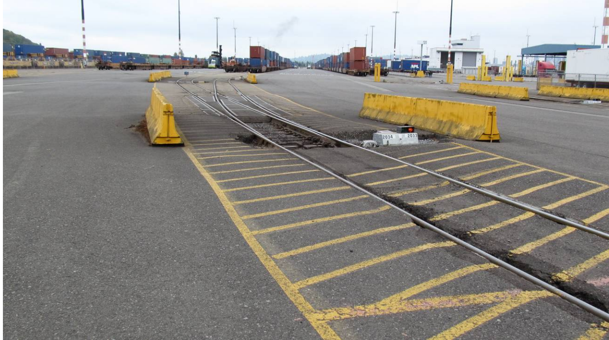
Photo 3: Asphalt Condition in Vicinity of Rail Lines – from the south
