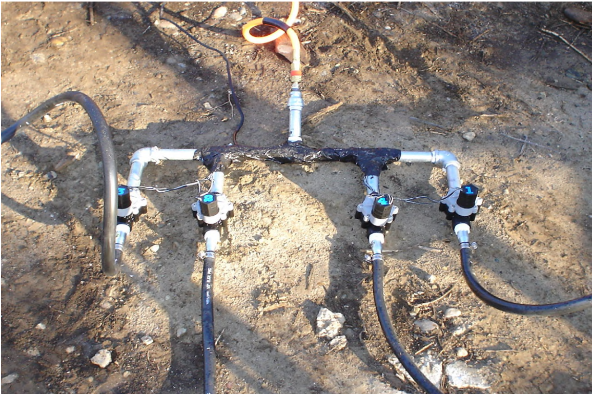
Air injection manifold.
