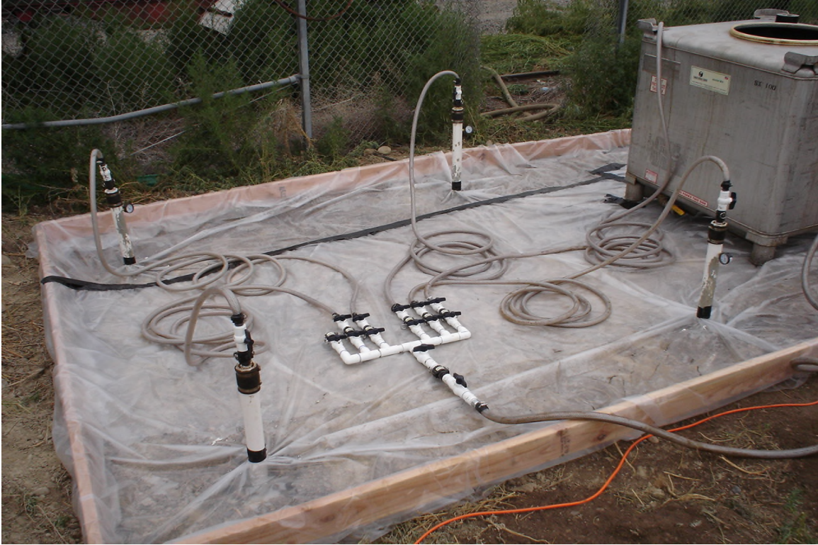
Manifold for delivery of sodium acetate solution to injection wells.
