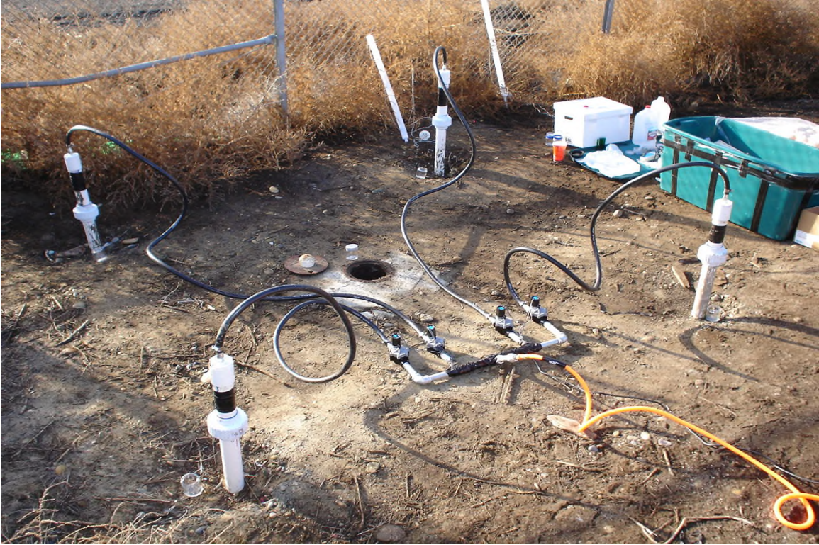
Air injection system.
