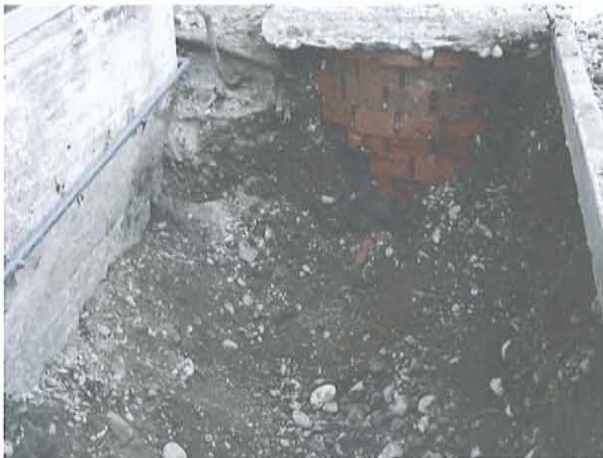
This view shows the drywell or French drain across the excavated area where the west tank was removed. This device is associated with the roof drainage system.
