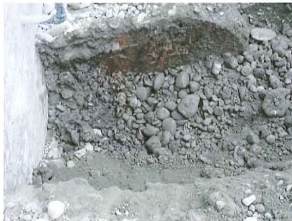
This picture shows the east end of the west tank. Notice the residuals of overfill and the large stones of the native material used for backfill.
