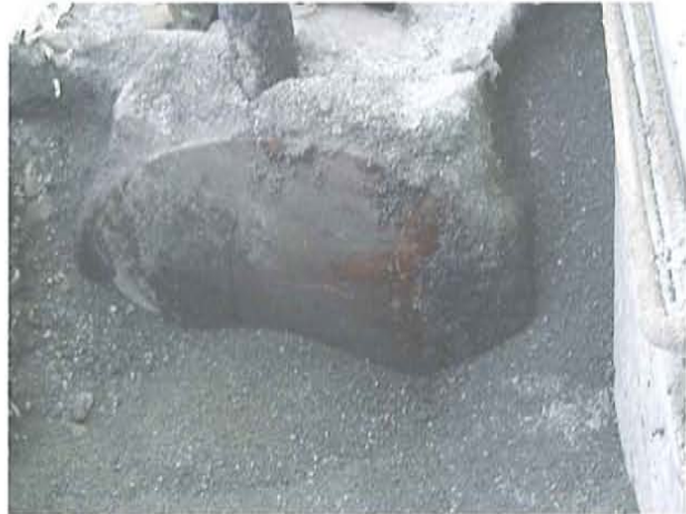
This picture shows the west end of the east tank. The overfill residuals are seen along the right side of the tank in the 3 o'clock position. Note the backfill.
