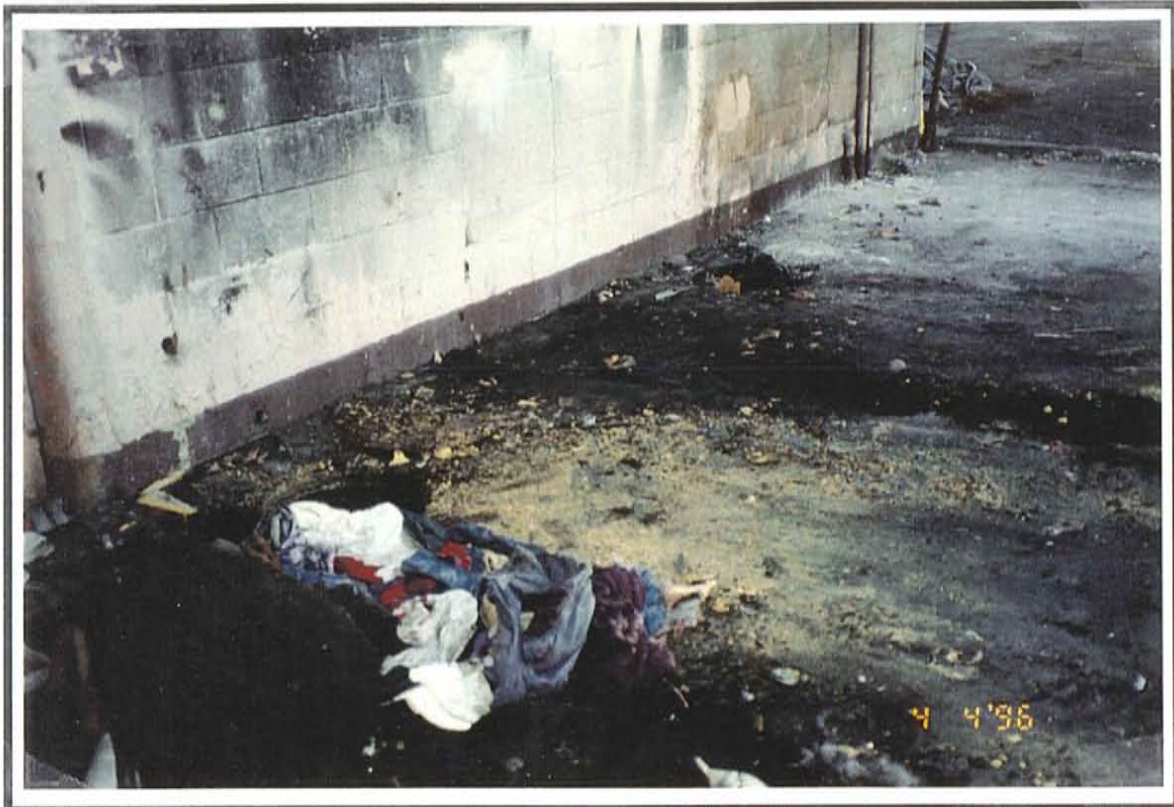
Photo 2. Two sumps along north wall of building (Sump #1 at left and Sump #2 at right).
