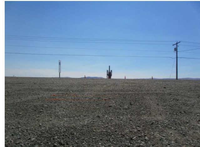
Drill rig positioned over MW-1. Photo taken at ground level facing South showing a significant crown over Vantage Highway
