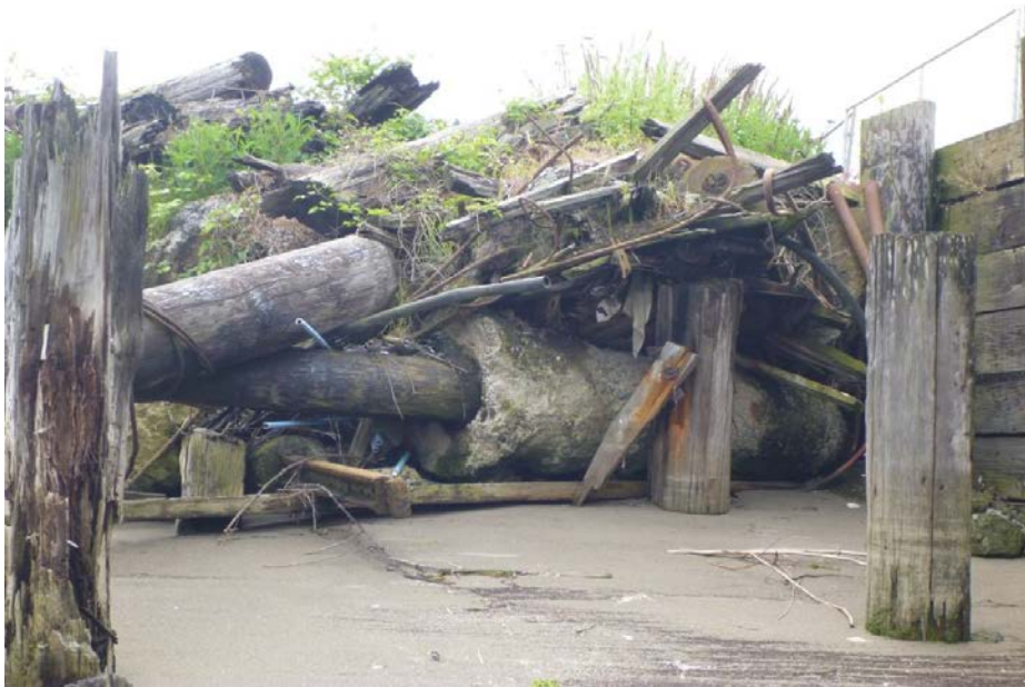
Plate 18 Manmade Shoreline Debris and Creosote-treated Timber Pile Stubs to be Removed, Southwest Corner of Log Pond Area (facing south)
