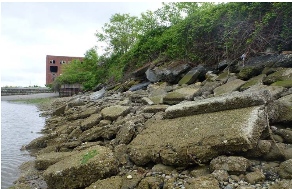
Plate 19 Concrete, Rebar, and Other Miscellaneous Manmade Debris to be Removed and Over-steepened Banks to be Capped along Central Portion of Log Pond Area Shoreline (facing east)
