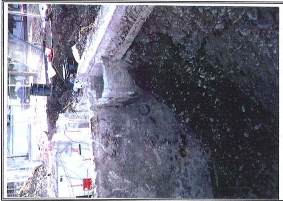
PHOTOGRAPHER: Rachel Tauman DATE: 10-12-94 VIEW: Excavation beneath the sump and old basement.
