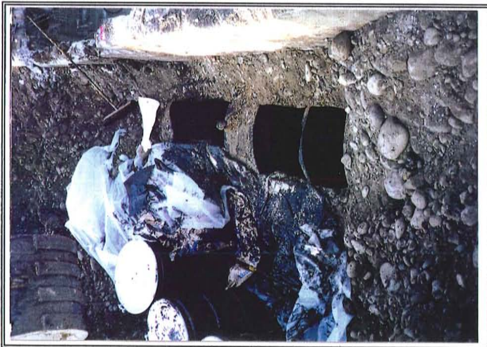
PHOTOGRAPHER: Rachel Tauman DATE: 10-12-94 VIEW: UST in the alley south of the sump.
