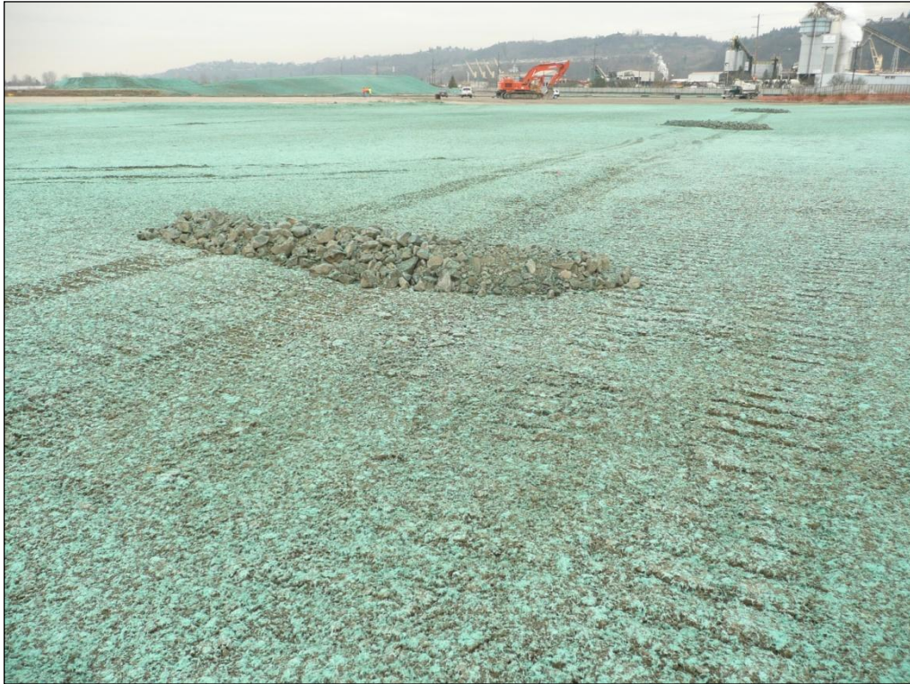
9. Looking northwest at the quarry spall check dams placed across the central drainage swale after completion of excavation backfilling.
