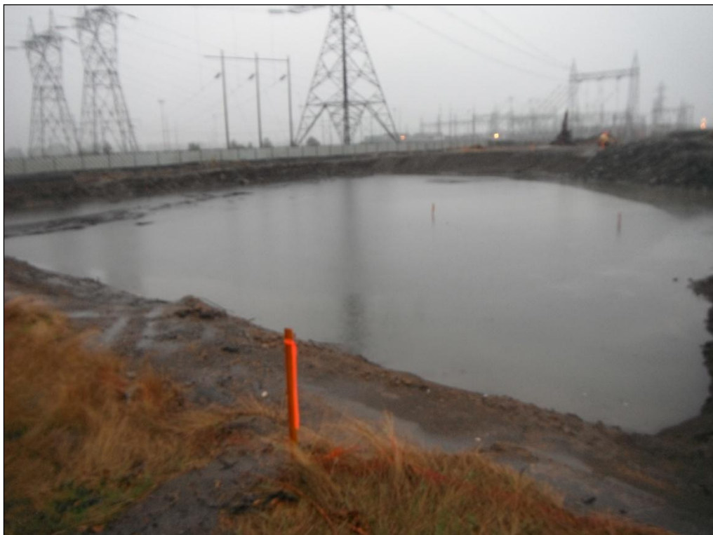
6. Looking southwest across the completed Closed Landfill excavation after a rise in groundwater level.
