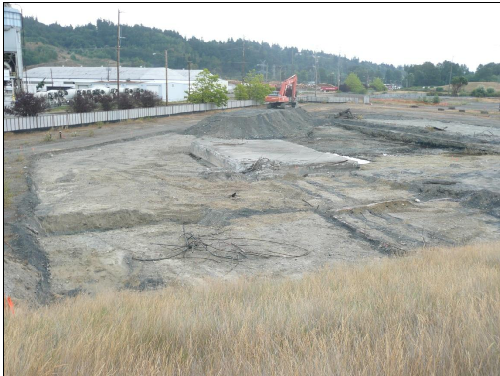
10. Looking southeast across the SPL Area excavation, with view of pot dumping slab, SPL material in utility trenches, and temporary stockpile of excavated SPL material to be loaded for disposal.
