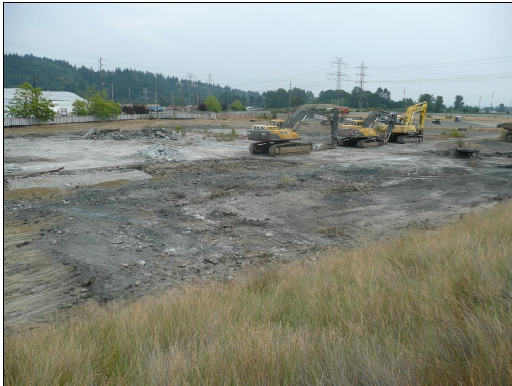
3. Looking southeast across the SPL Area during demolition of surficial concrete slabs and asphalt pavement.
