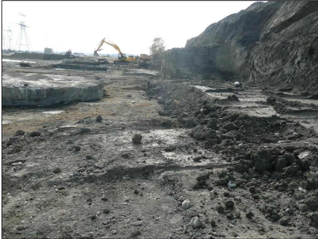
13. Looking south along the west side of the foundations of former buildings exposed during SPL material removal under the dredged soil stockpile.
