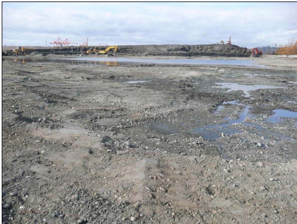
14. Looking west across the SPL Area excavation toward the dredged soil stockpile. Note water ponding in the deeper excavation areas.
