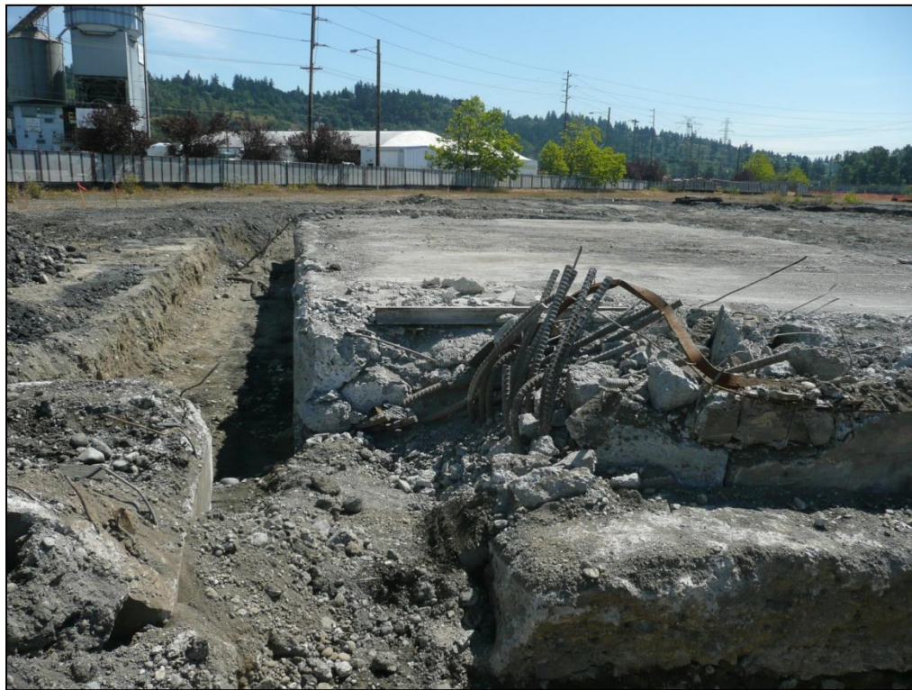
8. Close-up view of heavy rebar and steel rail reinforcement in the pot dumping slab.
