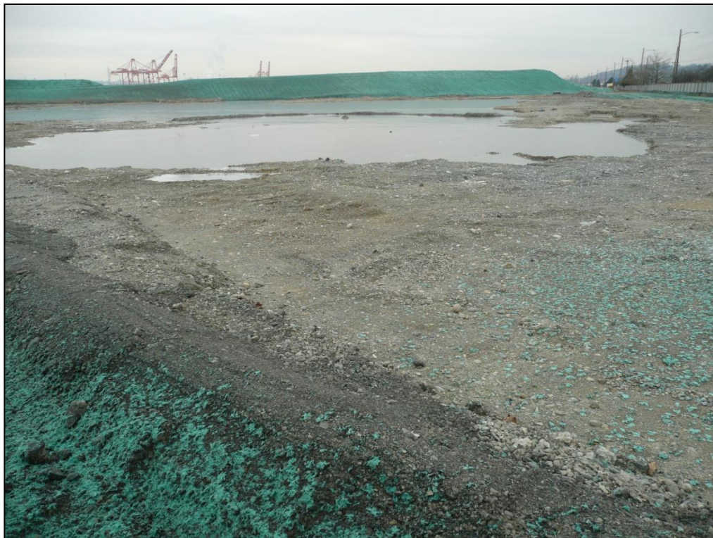
18. Looking northwest across the completed SPL Area excavation toward the dredged soil stockpile, with water ponded in a significant portion of the excavation.
