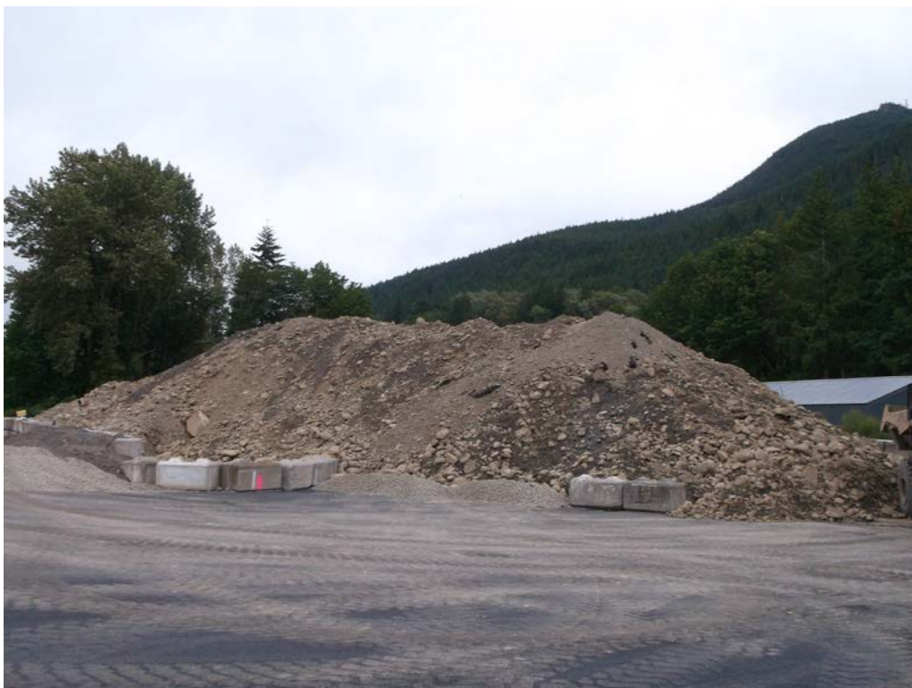
Photograph 12: Soil-handling facility, looking southeast.
