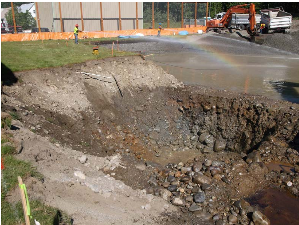
Photograph 8: Over-excavation in grid locations G10 and G11, looking west from grid location G12.
