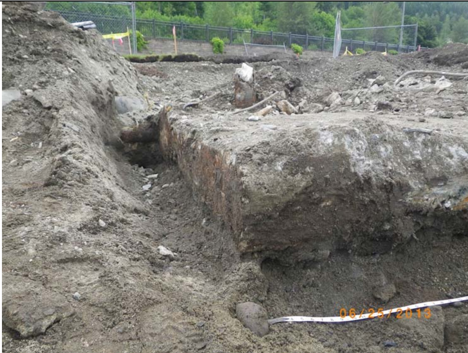
Photograph 3. View of southwest corner of foundation, showing remnants of wood cribbing (view to north-northeast). Also note vertical pipe (topped with ceramic, middle upper frame) and horizontal pipe extending from west foundation wall.
