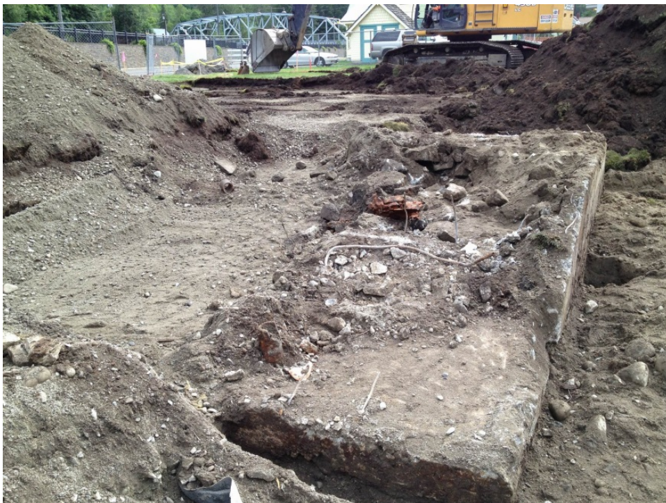
Photograph 2. View east-northeast of foundation, showing rubble in fill. Note vertical pipe to the northwest corner of the concrete foundation base.
