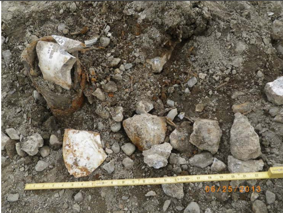
Photograph 9. Overview of vertical pipe and metal concentration to the east (note sanitary porcelain fragments). Ruler at 22 inches.
