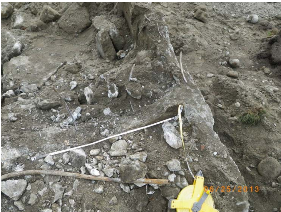
Photograph 4. View of outer (south) wall of foundation (right) with inner wall extending north (aligned with tape). View to southeast. Note rebar spaced along upper portion of concrete wall.
