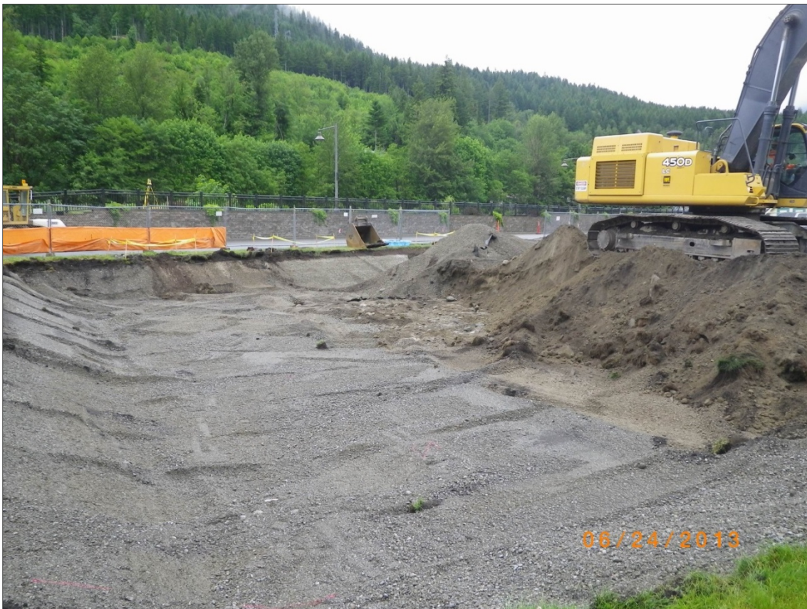
Figure 5-3. Overview of overburden excavations at the northwest portion of the AI, showing the transition from gravelly fill associated with the 2010 Levee Remediation to the yellowish-brown, siltier sandy and cobbly overburden and fill observed elsewhere (view to north).
