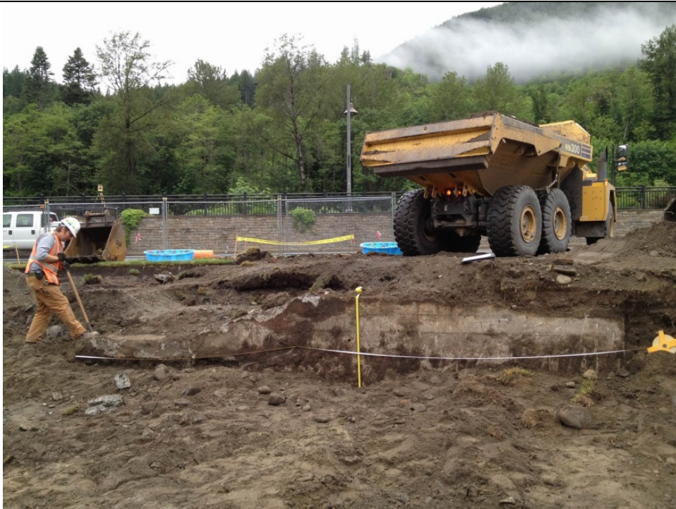
Photograph 5. View north of the south wall of foundation. Western 7 ½ ft is comprised of a concrete pad overlying packed sediments, while the remaining portion of the foundation consists of poured courses.
