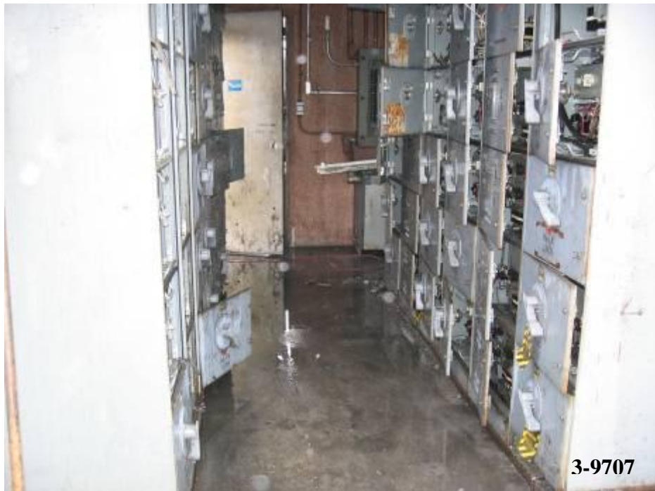
6.38 - Motor Control Center after final cleaning
