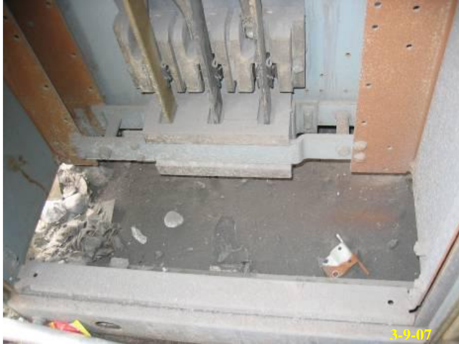
6.9 - Inside of main MCC breaker panel prior to cleaning
