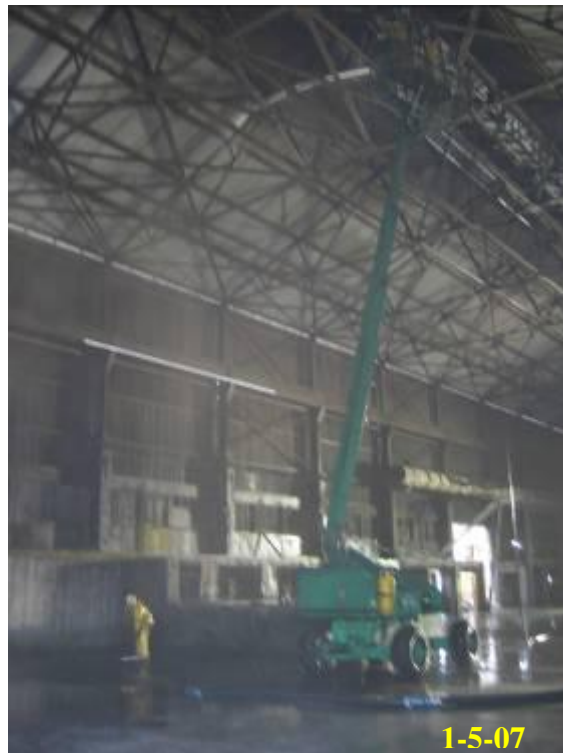
6.20 - Washing of building structure from manlift; Vacuuming of wash water from floor
