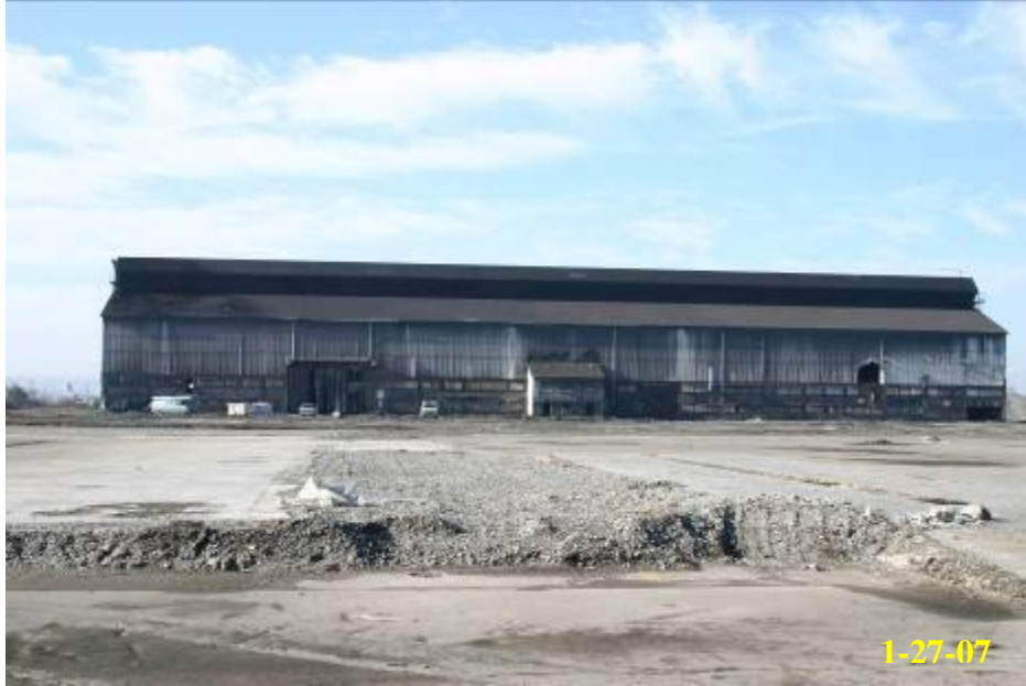
6.0 - East side of Building 65 prior to demolition; also shows encapsulant sprayed roof
