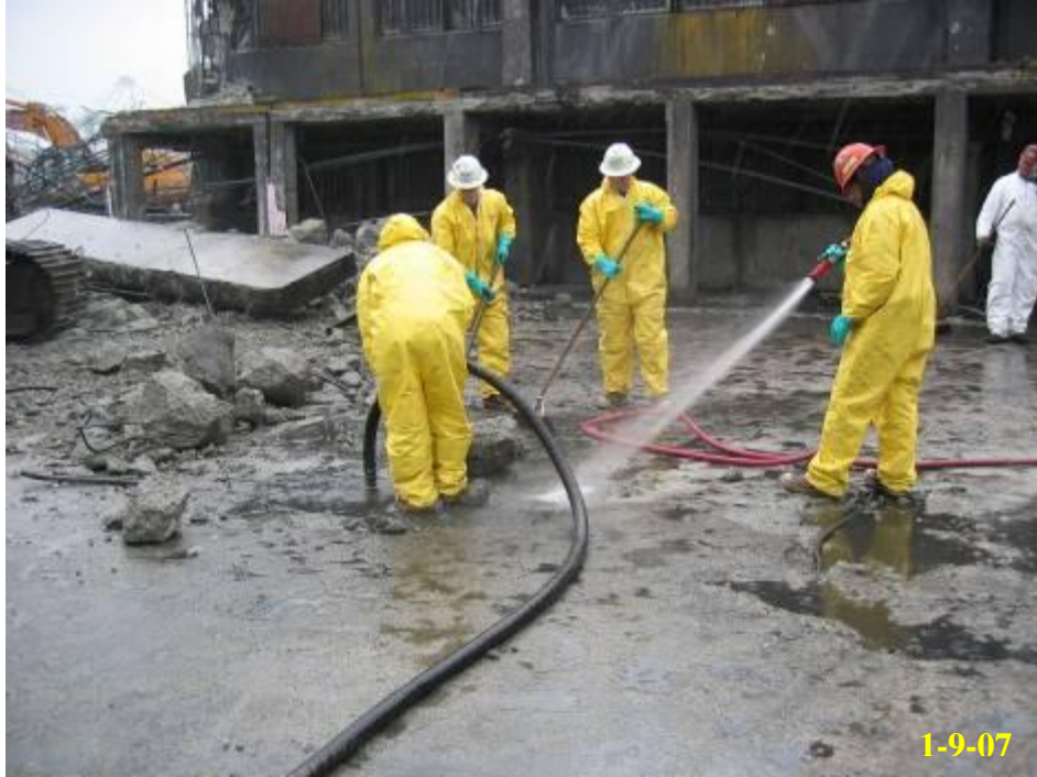
6.29 - Final washing of building floor after demolition of main metal portion of the building
