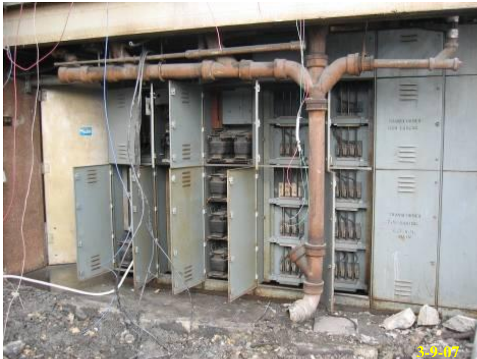
6.14 - Main breaker panels during cleanup
