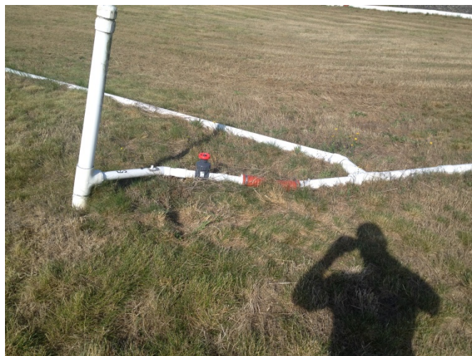
E27 after valve replacement.
