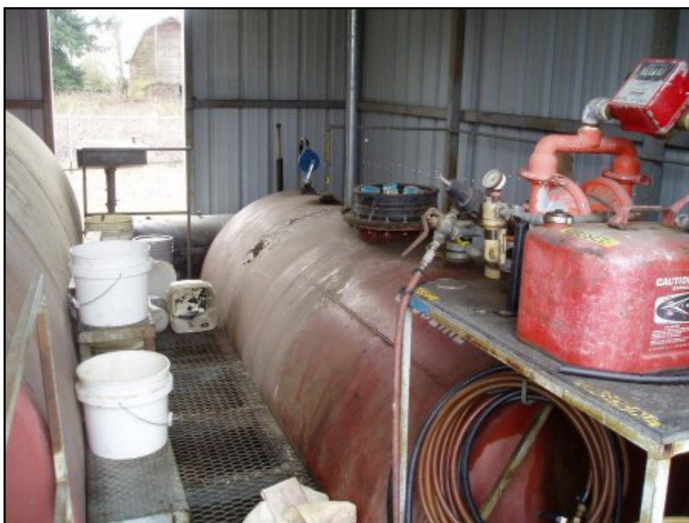
View of the 5,000-gallon gasoline AST located northeast of Building 14.
