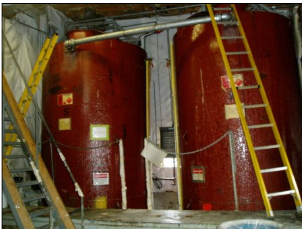
View of two 10,000-gallon resin tanks observed north of Building 2.
