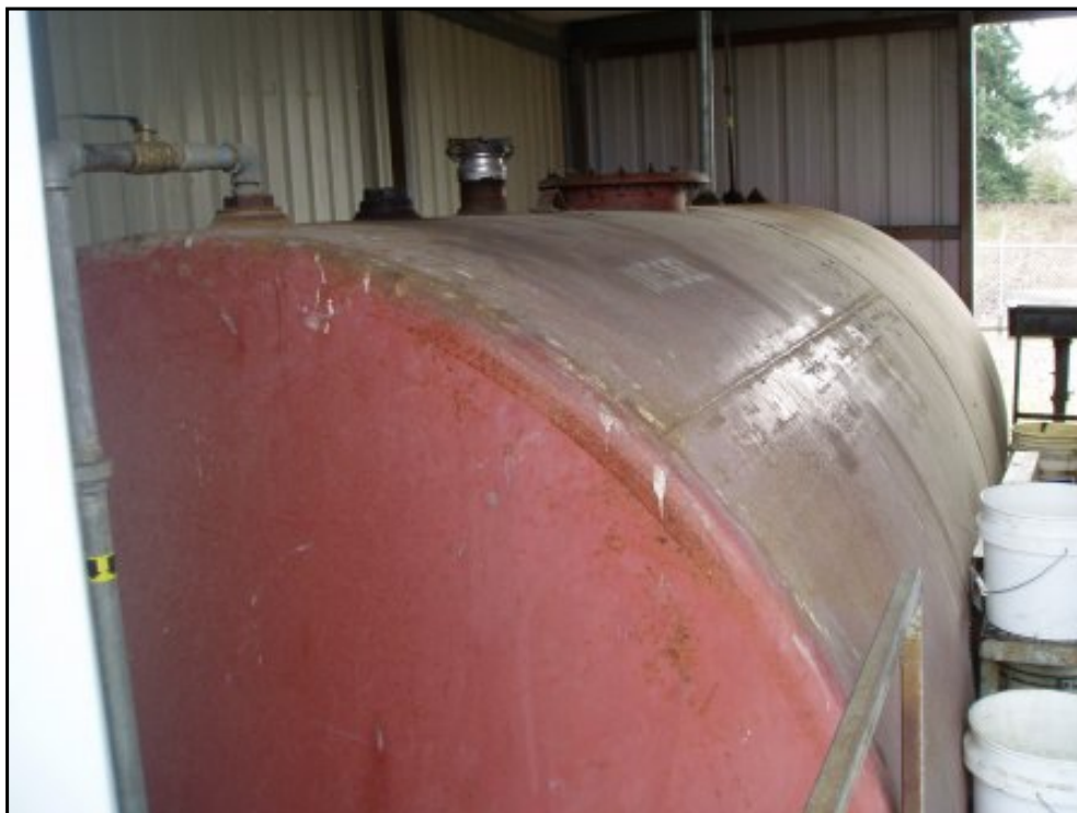
View of the 10,000-gallon diesel AST located northeast of Building 14.
