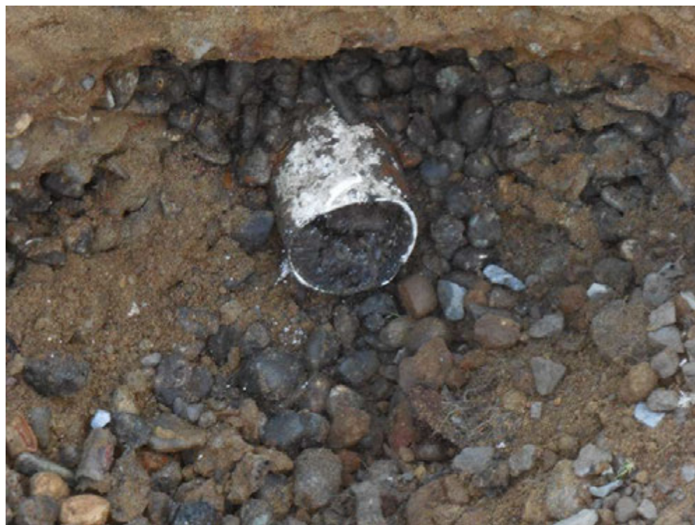
Photograph 4: Black substance inside perforated drainpipe.
