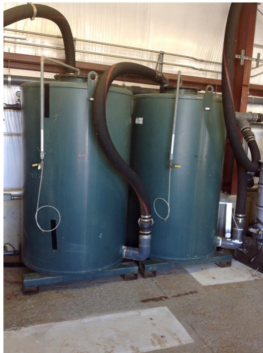
Photo 4: carbon treatment tanks (part of groundwater extraction treatment system)
