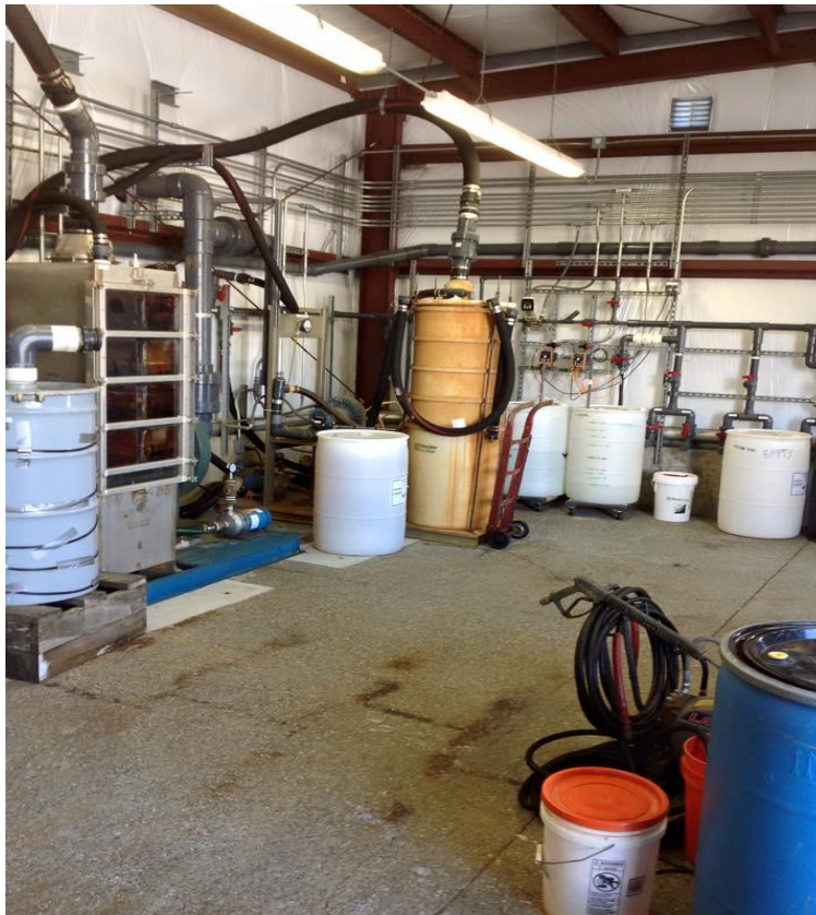
Photo 5: groundwater extraction treatment system (air stripper and [cylindrical, light-brown backup stripper])
