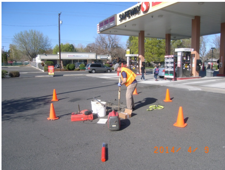
Advancing boring EB1A using a slide hammer and manual direct-push technology (DPT) - view north.
