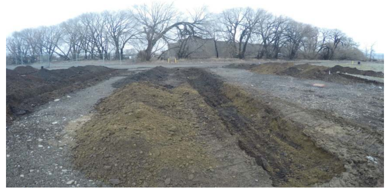
In this photo, inconsistent soil coloring can be seen indicating that the top foot or so of soil is not native.
