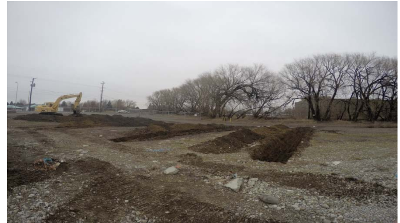
Trenches A through E (right to left) advanced near the former mechanic shop.
