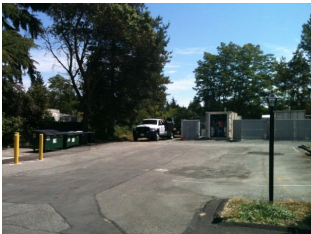
Photograph 17. The Drake and TOC/Farmasonis remediation systems conex, facing east on the TOC/Farmasonis Property.
