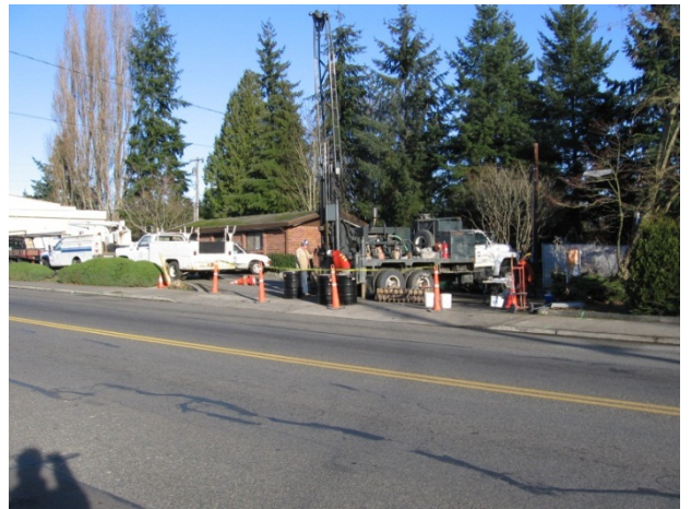
Photograph 10. Hollow-stem auger drilling on the TOC Property, facing east across 56 th Avenue West.
