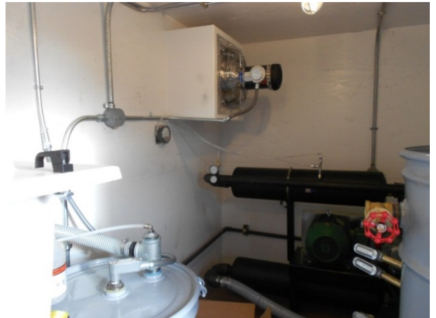
Photograph 18. A partial interior view of the remediation system housed in the conex box.
