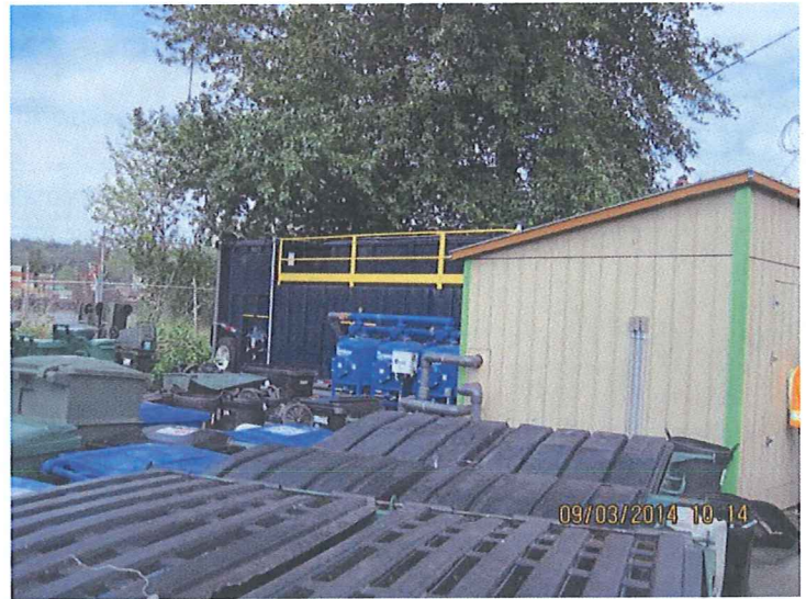
#4. DESCRIPTION: The dark blue tank is main stormwater treatment system for the majority of the site.
