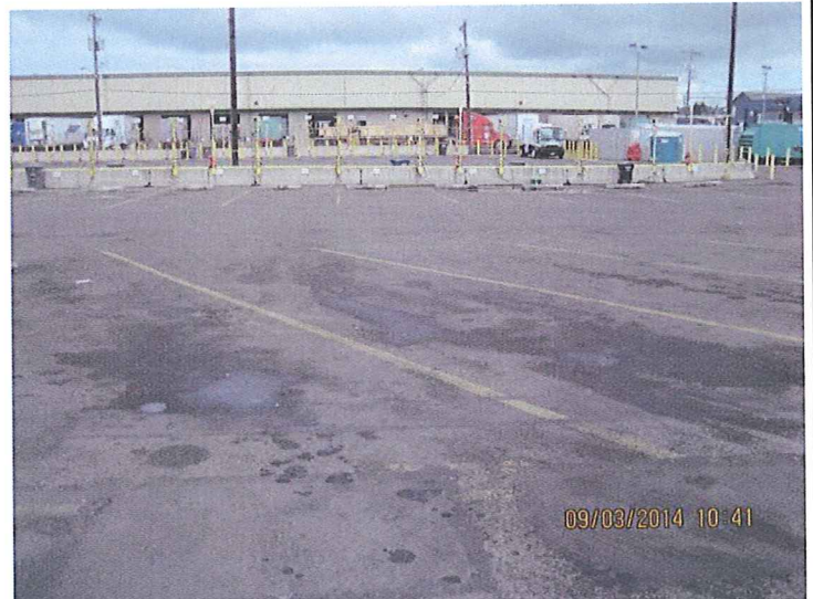
#12. DESCRIPTION: The amount oil drips and leaks were very noticeable. The permit requires the inspection of all equipment and vehicles during monthly site inspections for leaking fluids such as oil, antifreeze, etc. Take leaking equipment and vehicles out of service or prevent leaks from spilling on the ground until repaired. And immediately clean up spills and leaks (e.g., using absorbents, vacuuming, etc.) to prevent the discharge of pollutants
