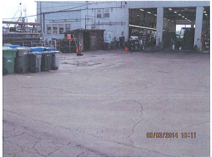
#2. DESCRIPTION: The facility must make sure that no process wastewater generated from equipment and/or truck maintenance activities can flow to the storm drainage system. This area is bermed and flows to the sanitary sewer.
